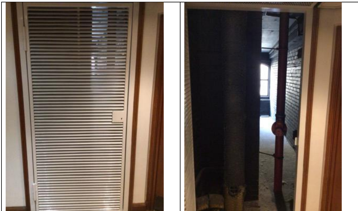
Figure 4 - Smoke Shaft Door
