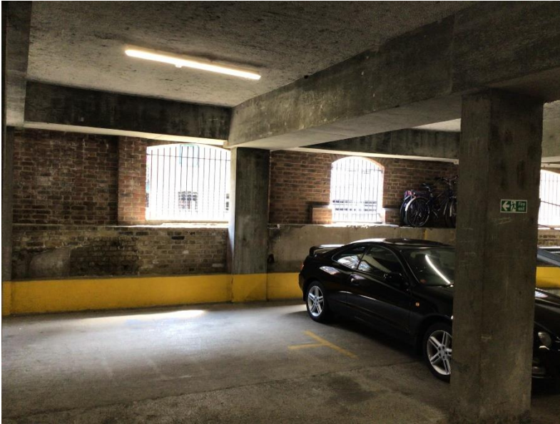
Figure 2 - Natural Smoke Vents Within Car Park - River side
