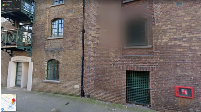
Figure 3 - Dry Riser Inlet Position
