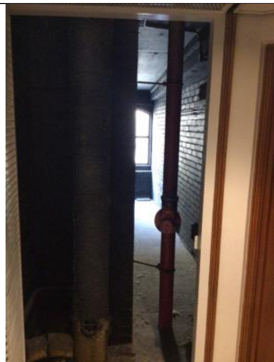
Figure 5 - Dry Riser Location Within Smoke Shaft
