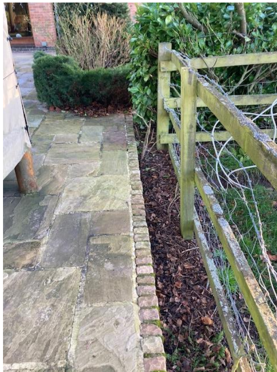
12. Rear south west side paving edge and timber fence to the grass paddock.
