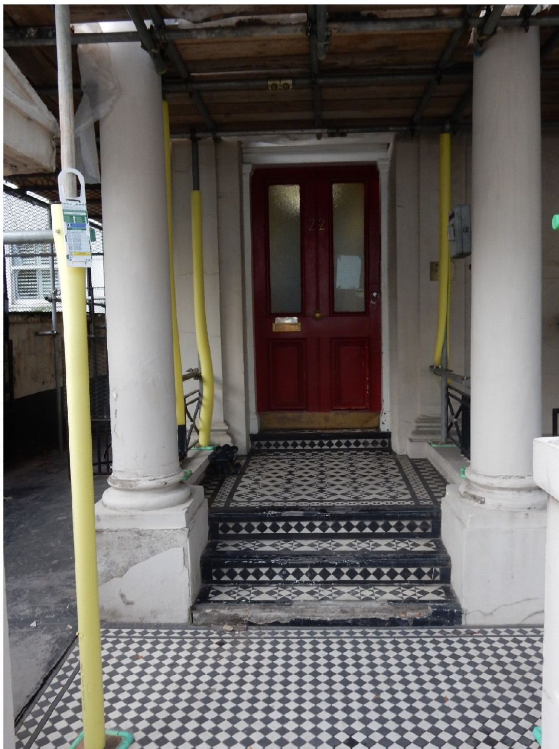
Above: Existing run-down Victorian style black and white tiles.
