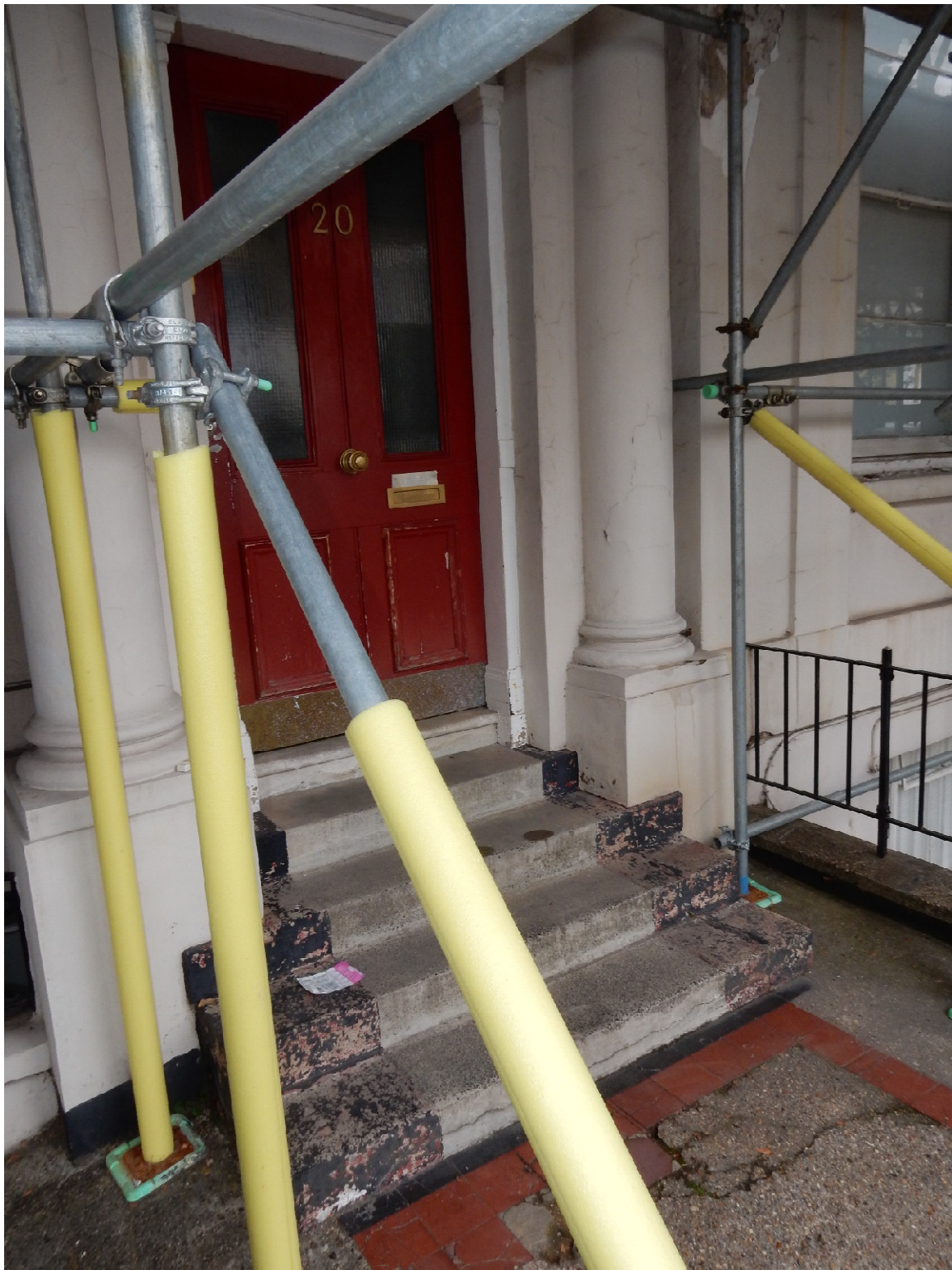
Above: Existing dilapidated front entrance steps and surface finish to No.20 terrace.
