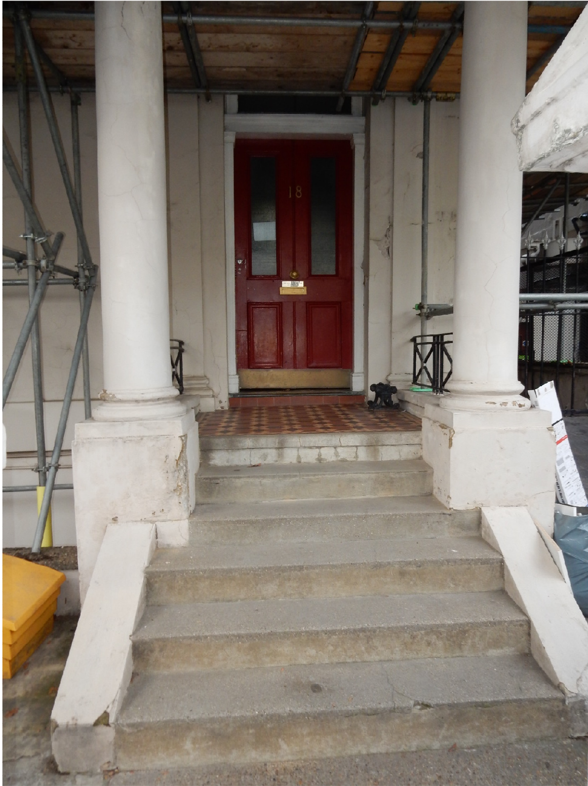
Above: Existing dilapidated concrete front entrance steps and surface finish to No.18 terrace.
