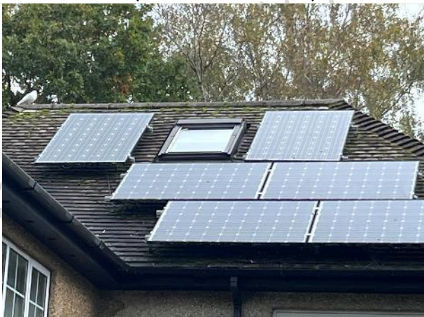
External Feature: roof tiles and ridge tiles at the rear elevation of the upper floor with low potential for bat access
