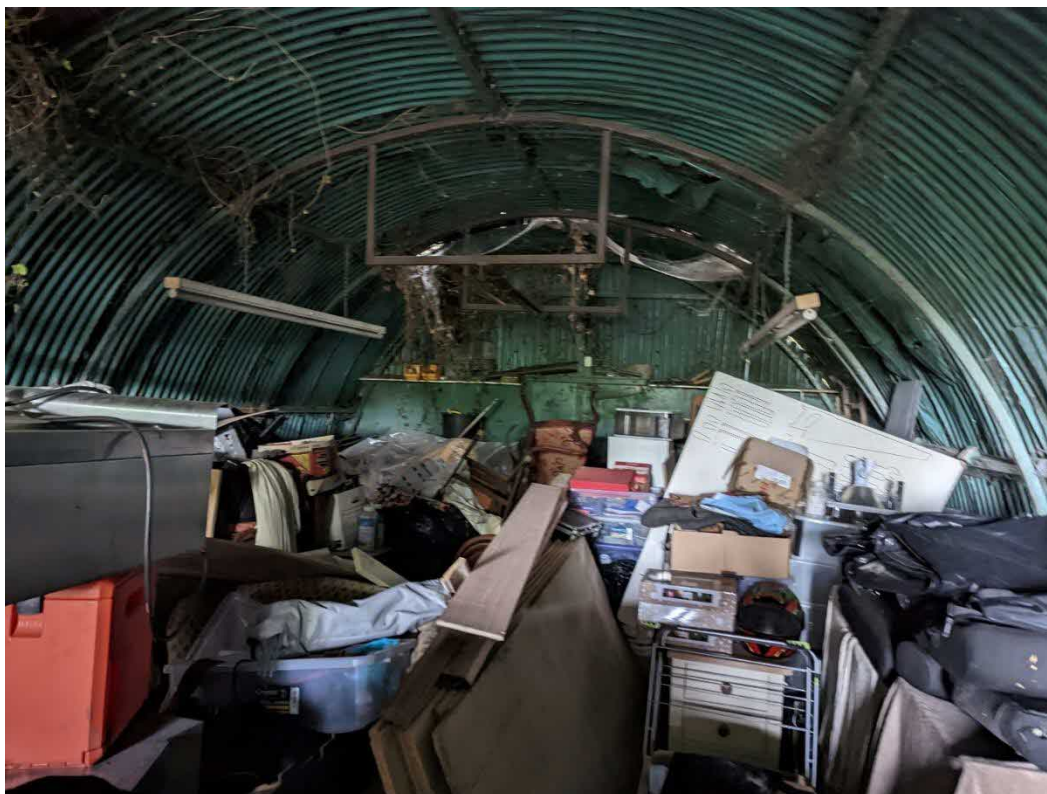
Internal view of Nissen Hut, showing the curved structural T-Shaped ribs, purlins and corrugated Iron sheeting exterior.
