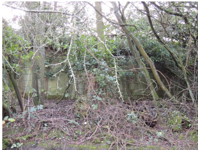
Photo 14: The north-western elevation is obscured by Ivy
