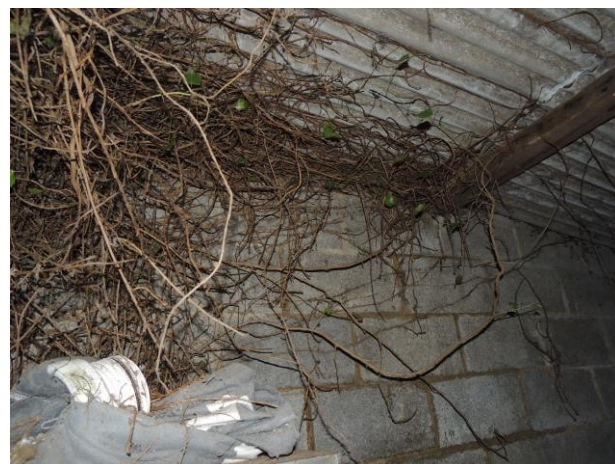
Photo 3: Note Ivy growing into the building
