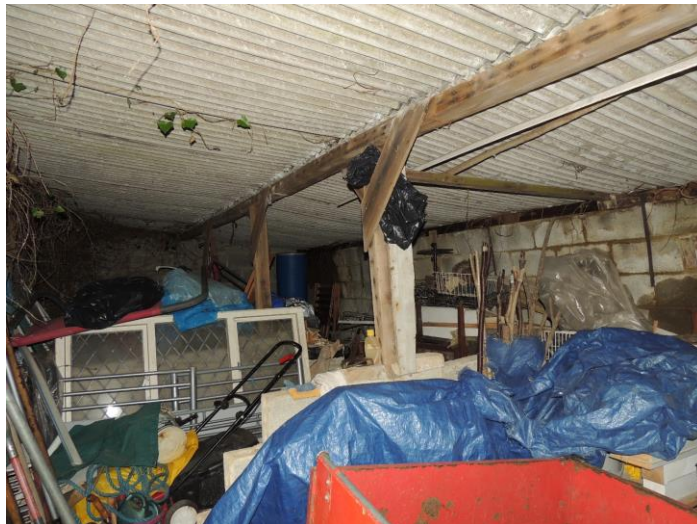
Photo 7: Interior of the building. Note lack of features that might be occupied by bats
