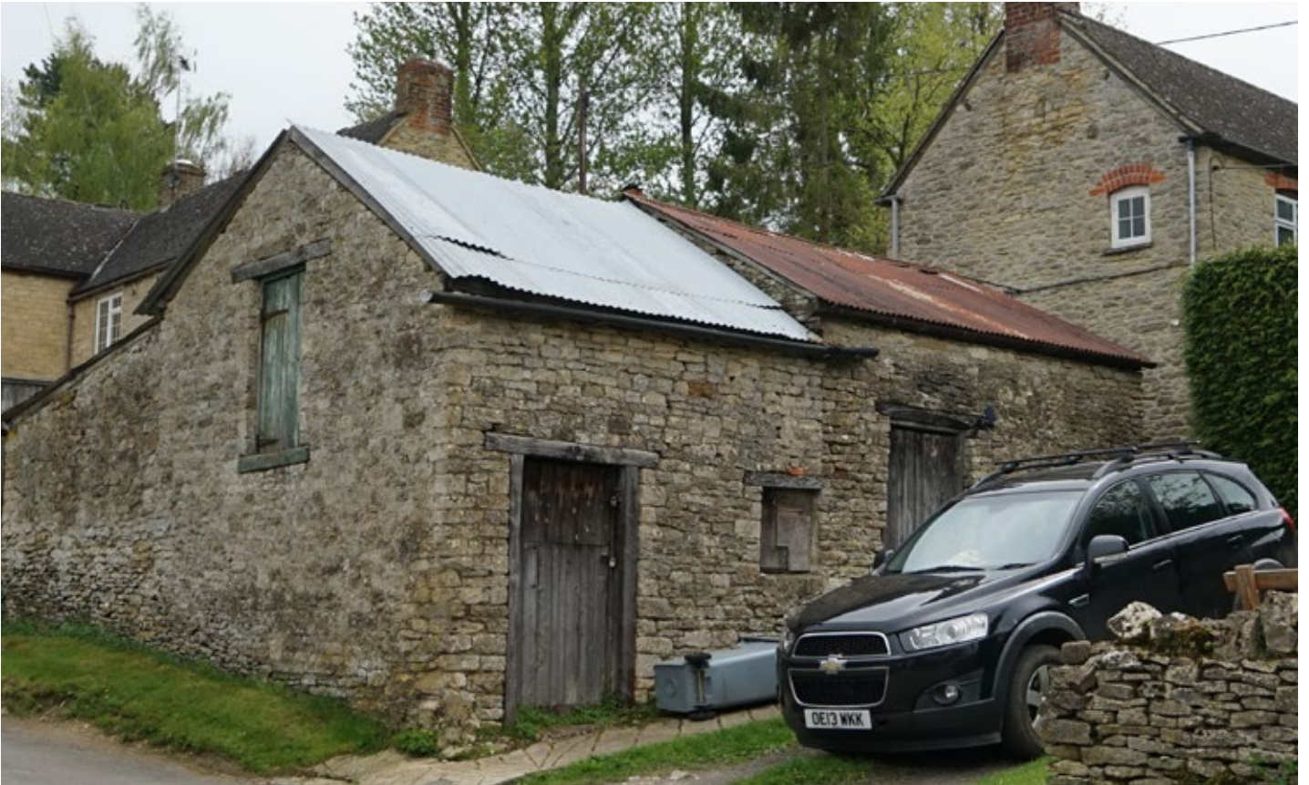
View of the two former stables. The one nearest the house slightly higher with a slacker pitch under a rusty corrugated iron roof is the earlier range. The stable to the roadside has a slighter steeper pitched roof, also in corrugated iron and is the later building, possibly early 20th century. Notice the clear straight joint between the two. The lean-to to the rear appears to have been built above an existing boundary wall to the road. Door to gable access a hay loft to the stable
