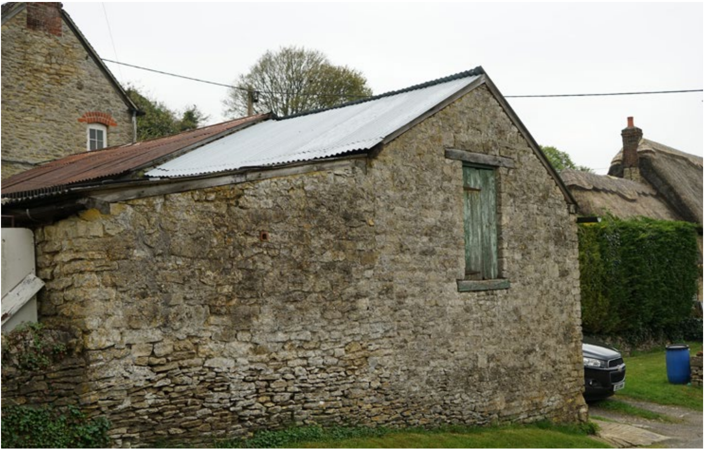
View showing detail of the changes in stone work between the lower and upper levels of the north wall
