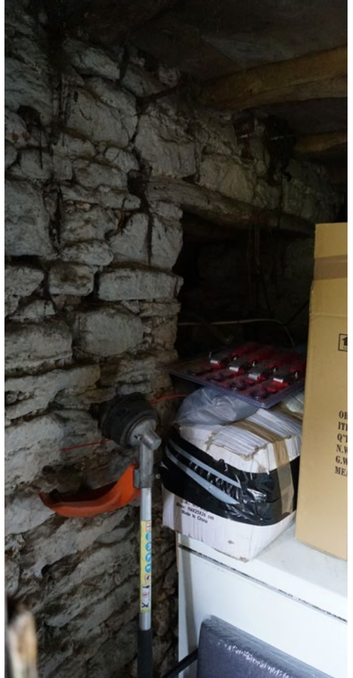
The north wall of the earlier range includes a former window opening, confirming the road-side range is a later addition
