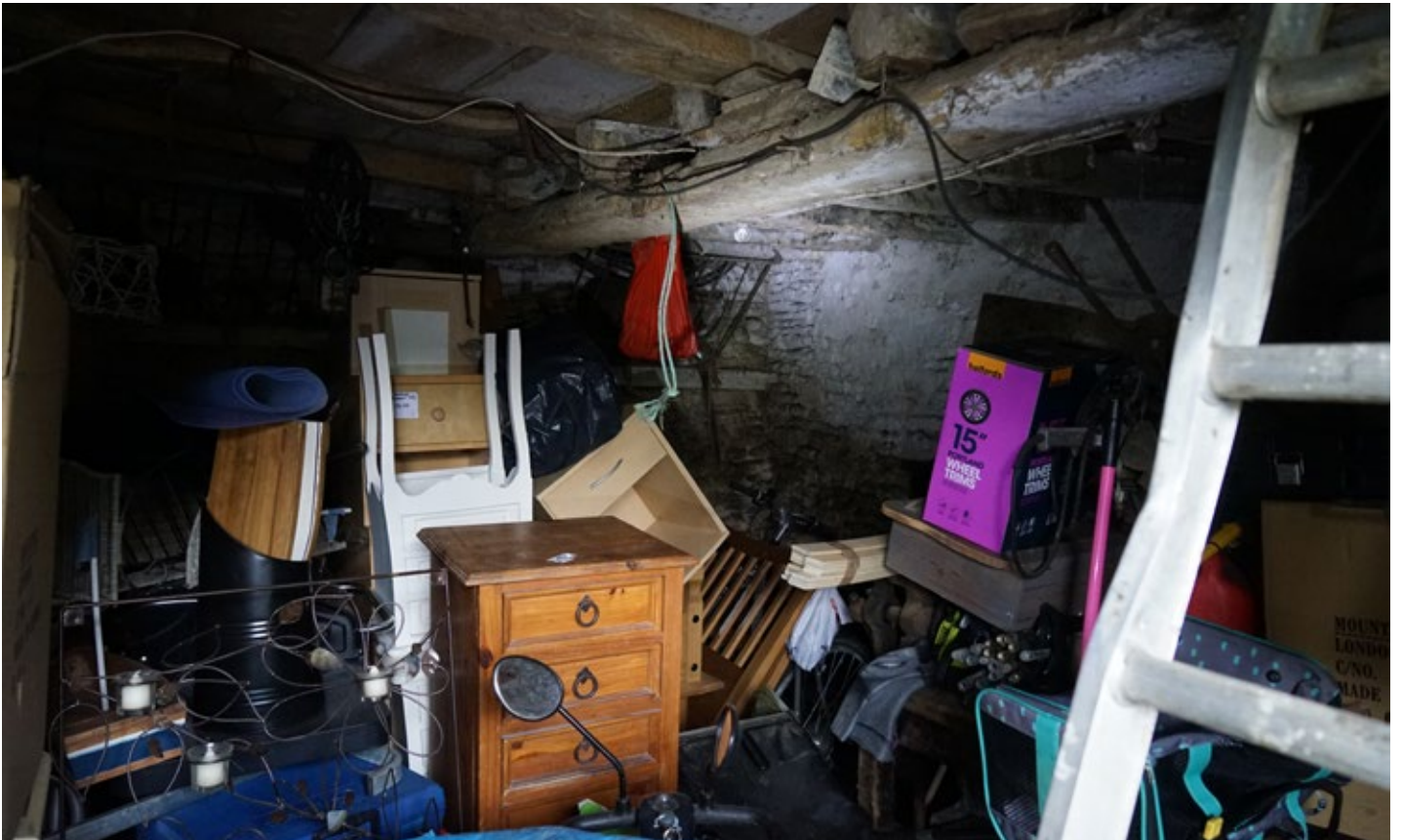
View of the ground floor of the southern (earlier) former stable showing timber floor structure with ladder to first floor
