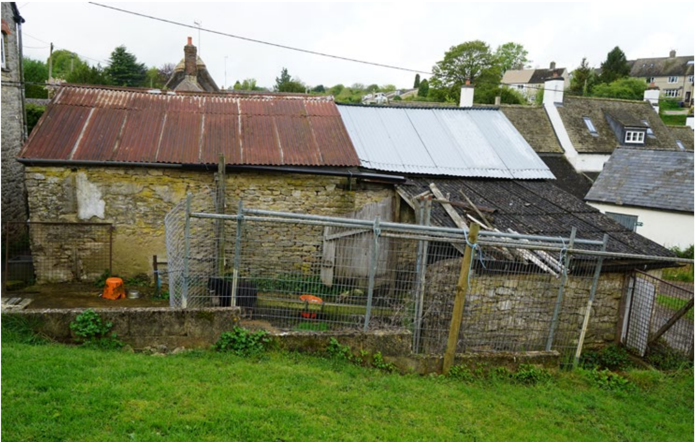
View of the stable range from the east showing the two ranges and the lean-to
