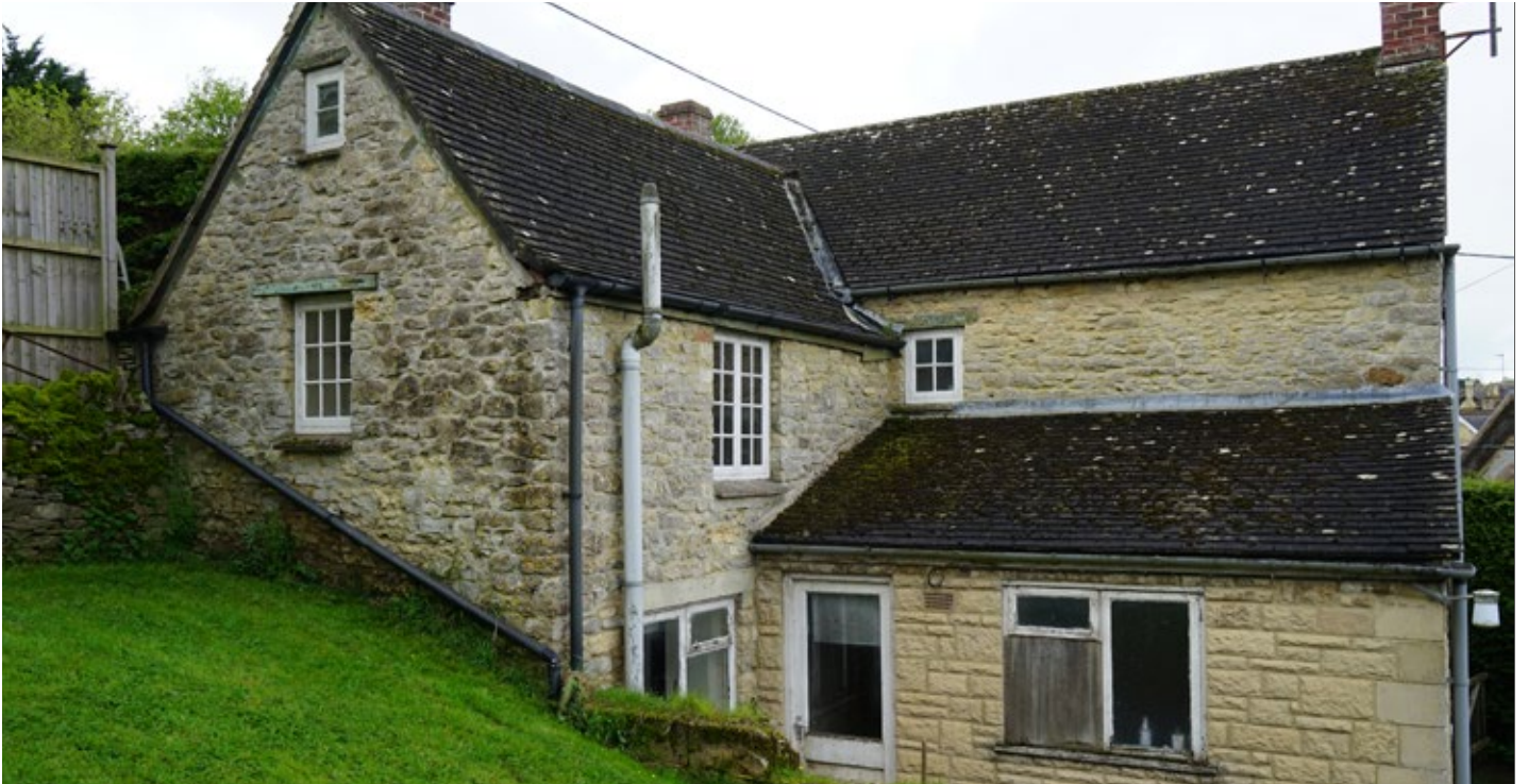
View from the east showing what is likely to be an earlier range, shown on the 1847 Tithe, with steeper pitched roof, timber heads to windows set hard against the southern boundary, with later range to the west and modern lean-to addition
