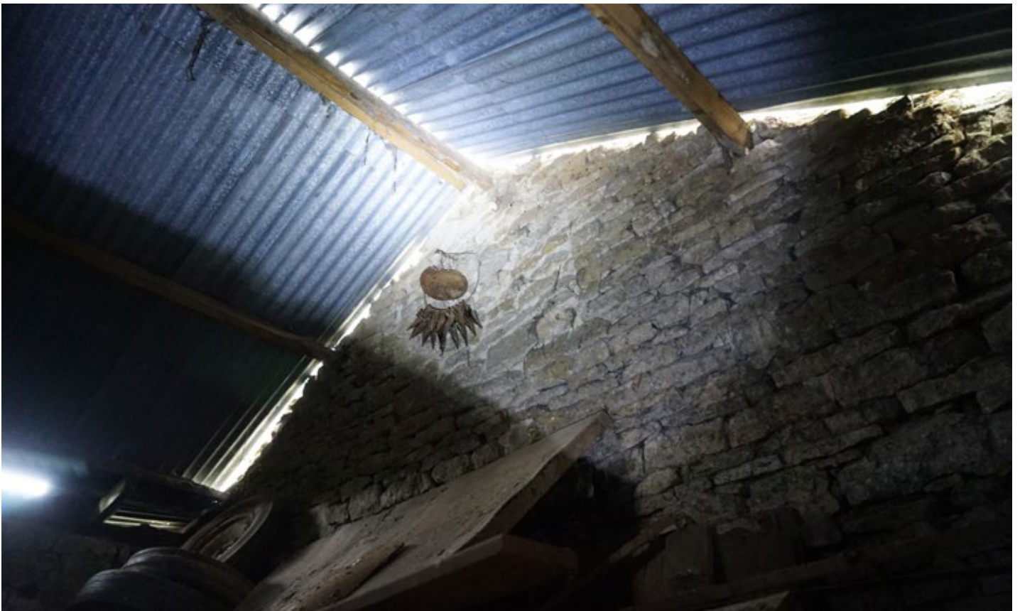
Roof structure to the northern stable building – modern timber ridge and single purlins
