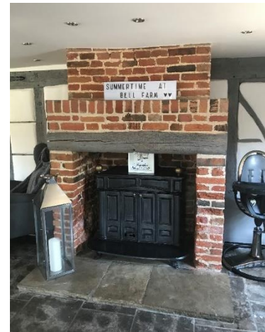
Figure 16 - Chimney stack at ground floor within the rear part of the house. Timber framing is visible in the internal wall behind.
