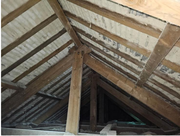
Photograph 3: Roof space interior showing detaching lime mortar
