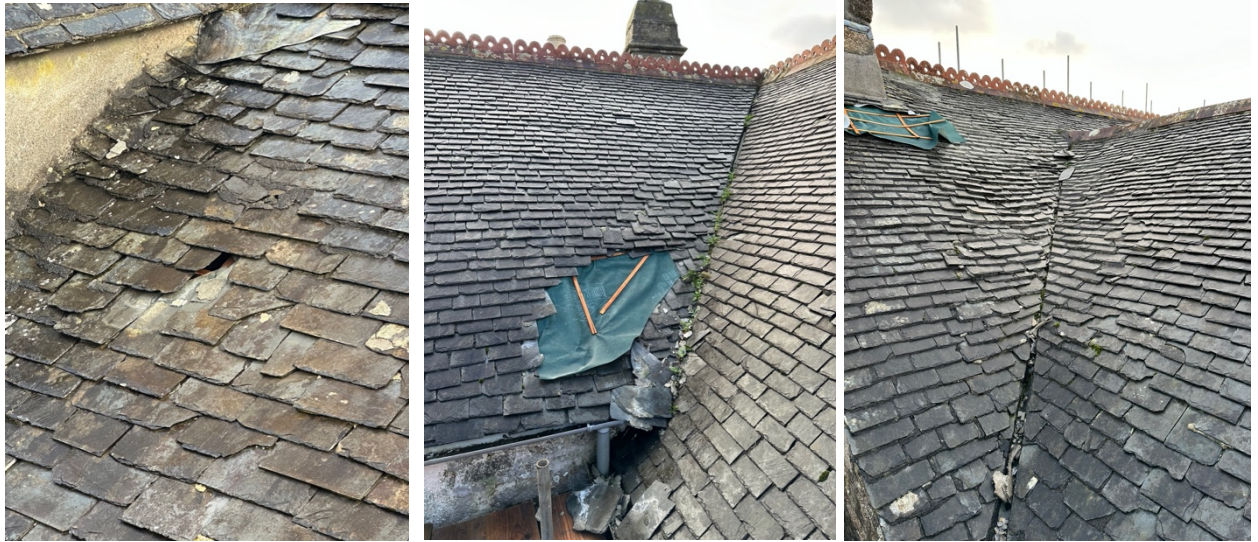
Figures 3-7 Recent roof damage following autumn storms
