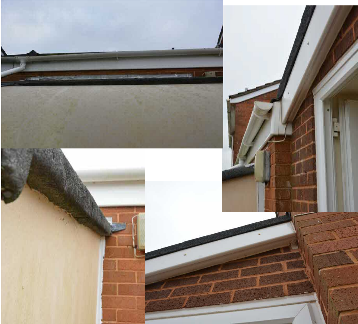
Figure 8:- Photographs illustrating the good state of repair of the features surrounding the garage and linking structure, which might usually offer potential access locations, to wildlife, into the buildings.
