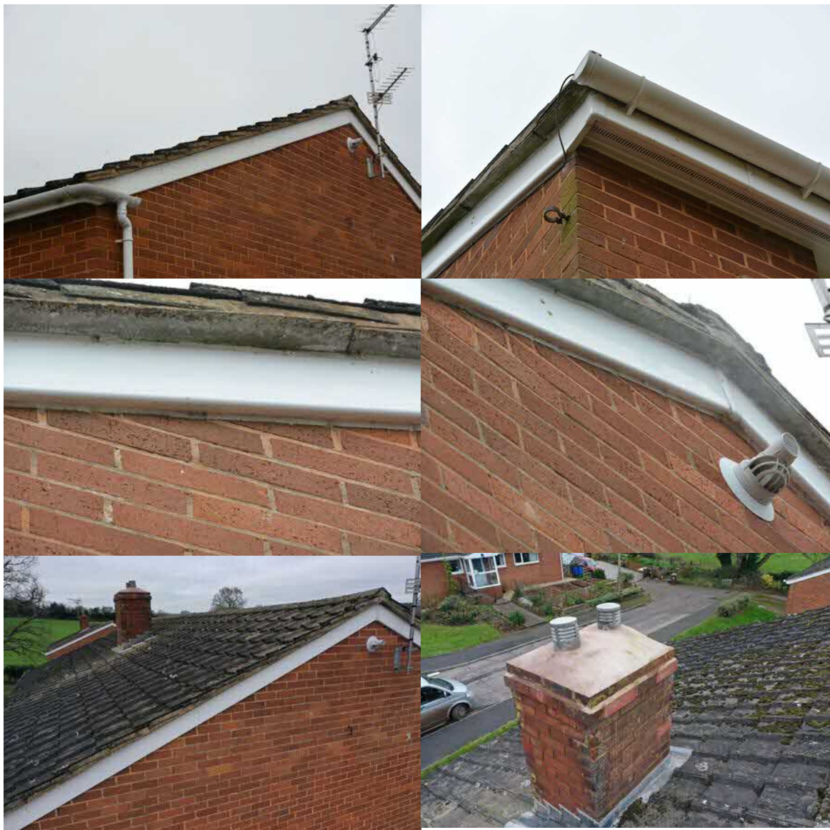
Figure 7:- Photographs illustrating the good state of repair of the features mentioned above in the text.
