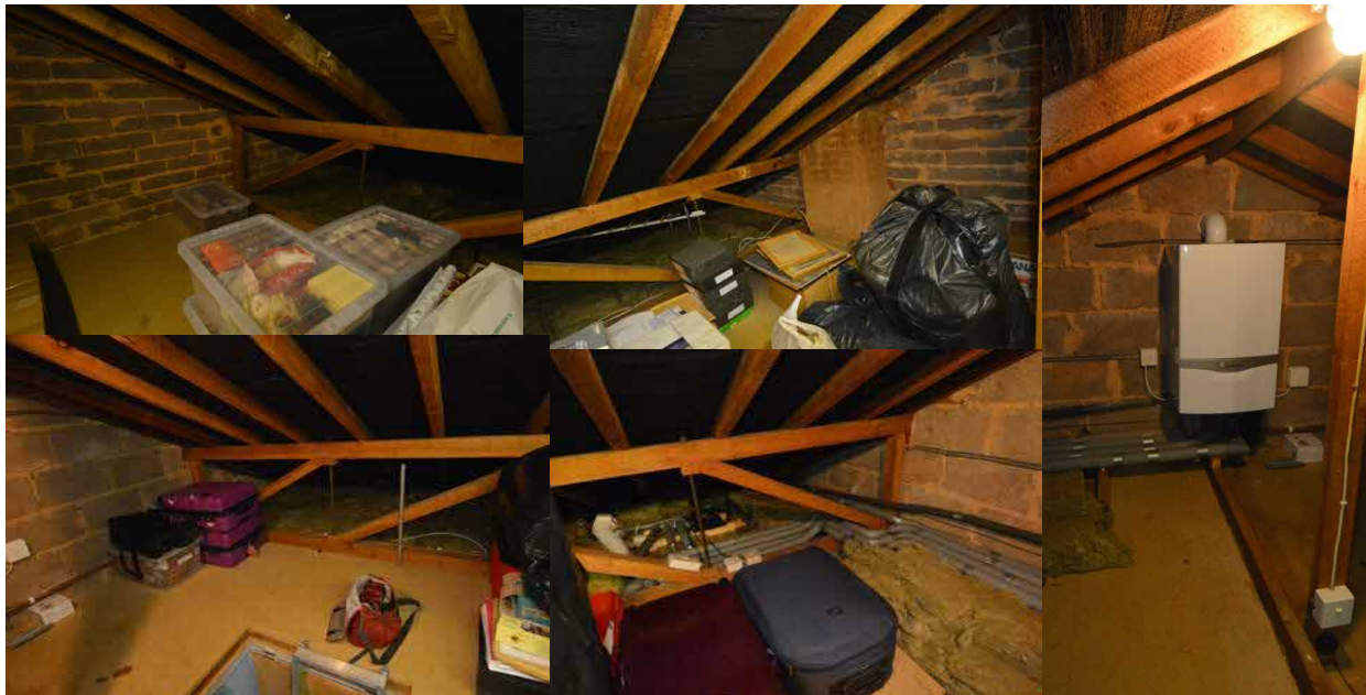
Figure 4:- Series of photographs illustrating the condition of the loft and its current use.
