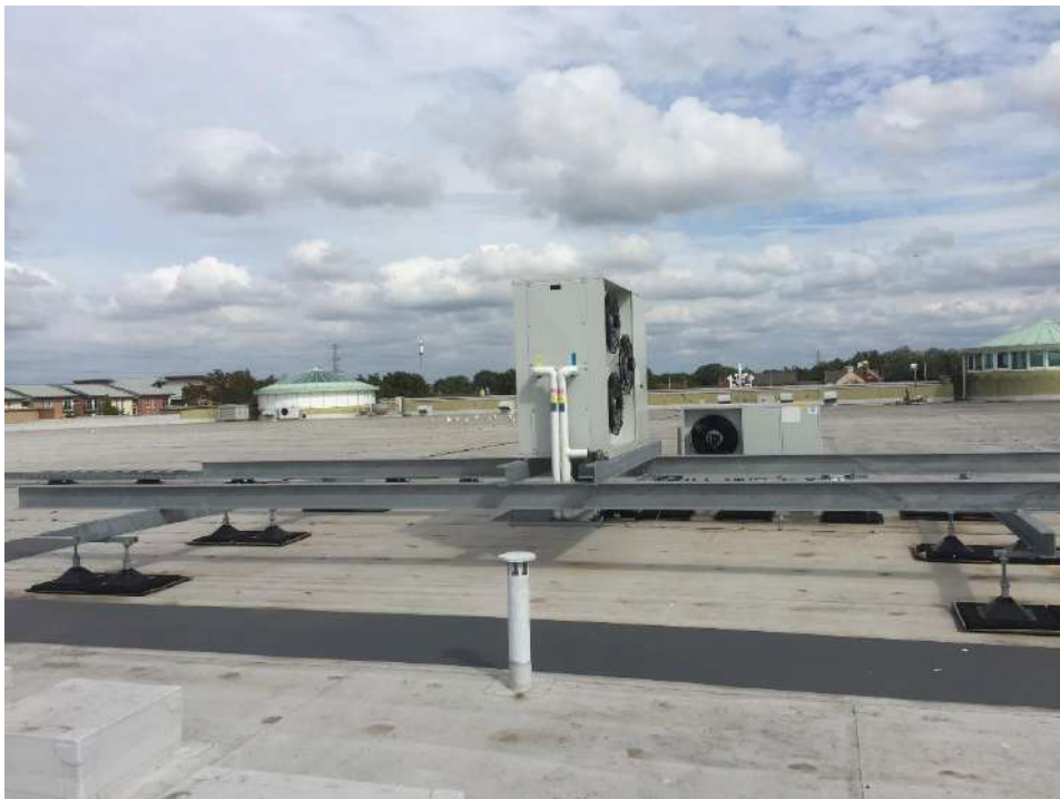
View looking North East across the roof from the roof over the warehouse area
