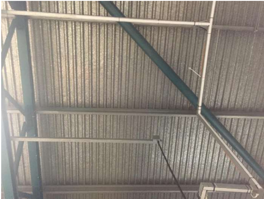
View on the underside of the roof decking and secondary lattice truss to the warehouse area
