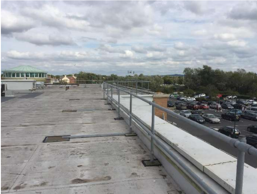
View looking North East along the rear of the South East parapet.
