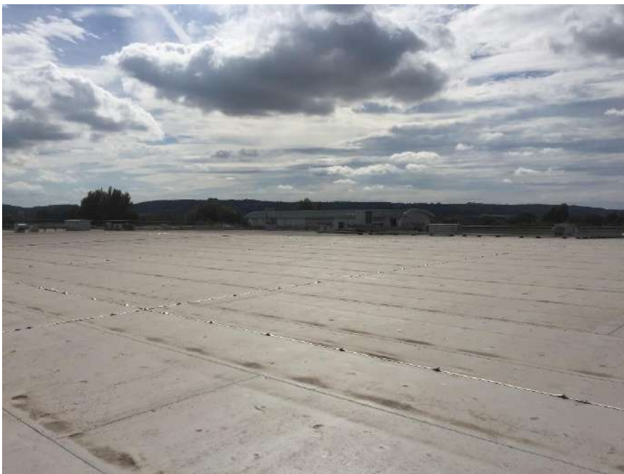
View looking South across the store roof towards the first floor plantroom & warehouse area
