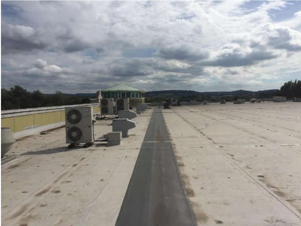
View along the rear of the North East parapet looking towards the Main Entrance area
