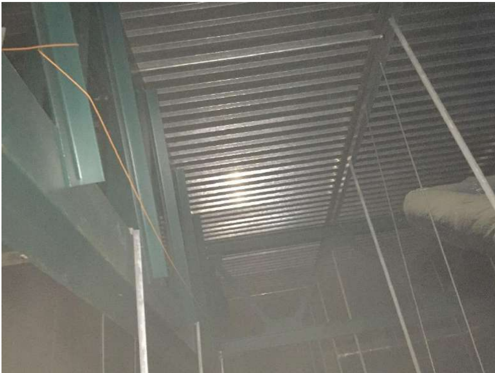
View along a spine truss seen above the ceiling in the store area
