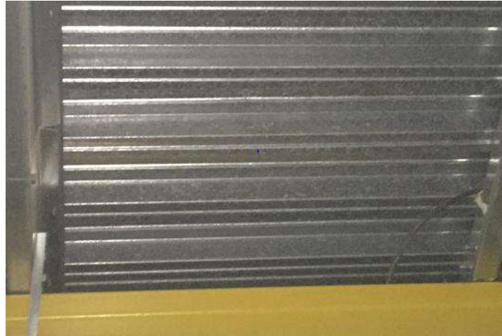
Figure 4 view on the underside of the roof deck in the store extension
