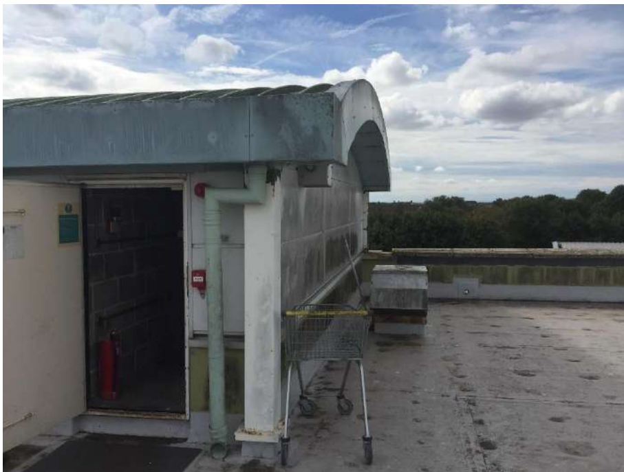
Shopping trolley left on the roof
