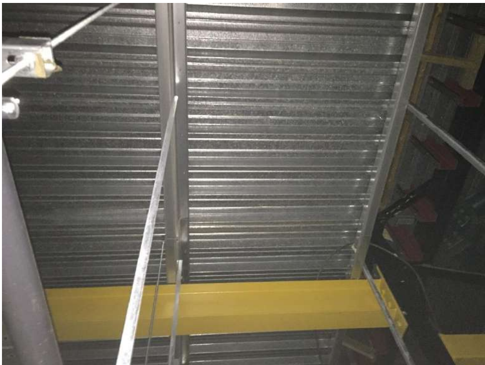
View on the underside of the roof decking and UB rafters in the store extension Seen above the ceiling in the store area
