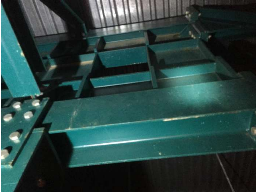
Fully plated end to a spine truss at the column connection, seen above the ceiling in the store area
