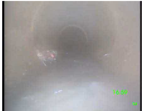
SMH1X_07097504-8e01-4bd2-a716-56a4448125cf_20231019_215657_698.jpg, 00:02:00, 16.59 m Roots, fine at joint
