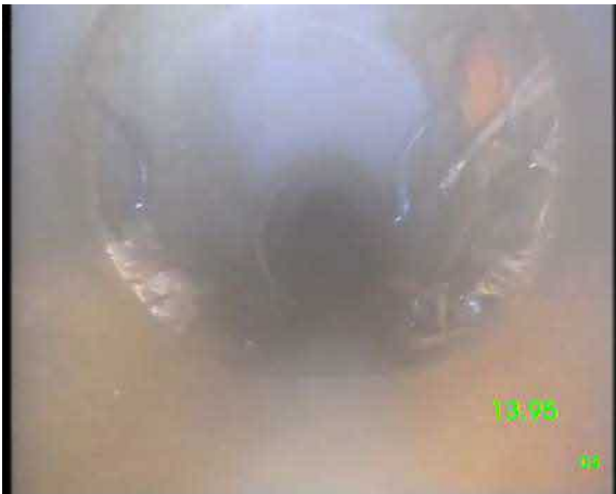
SMH1X_12570131-3300-499d-a56e-1378067cbf55_20231019_215628_599.jpg, 00:01:44, 13.95 m Roots, mass at joint, 25% cross-sectional area loss
