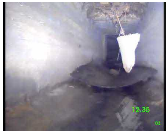
LINE AX_51119c05-b6b0-4d53-b790-fe8b2b8e773f_20231019_2204 16_451.jpg, 00:02:24, 12.35 m
