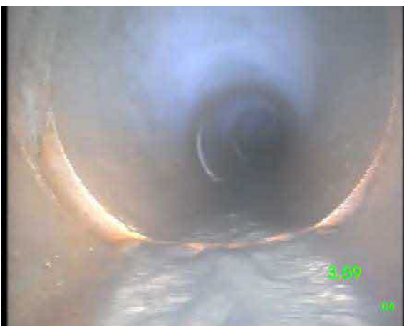
SMH1X_bec6f80d-dce7-4835-89f9-17849e65ee8d_20231019_215505_428.jpg, 00:00:40, 3.59 m Open joint, medium
