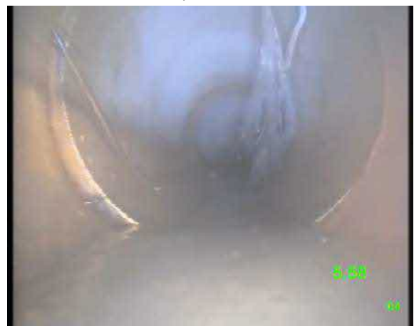
SMH1X_c18a7041-9d22-4cdb-b142-e95d9b6b8000_20231019_215525_810.jpg, 00:00:52, 5.58 m Roots, fine at joint
