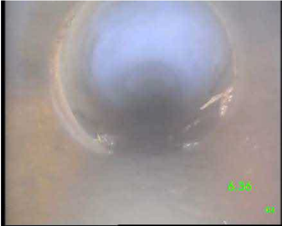
SMH1X_e1206aec-17cc-426f-8ea0-5966a2ee4935_20231019_215540_650.jpg, 00:00:58, 6.41 m Joint displaced, medium
