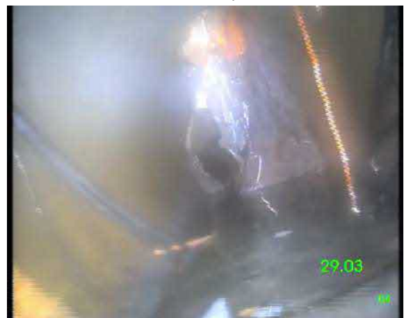
SMH1X_7f7a1bf8-934b-4edd-a8df-ee5f6865581c_20231019_215926_148.jpg, 00:03:14, 29.06 m Connection defective, blocked and intruding at 12 o'clock,
