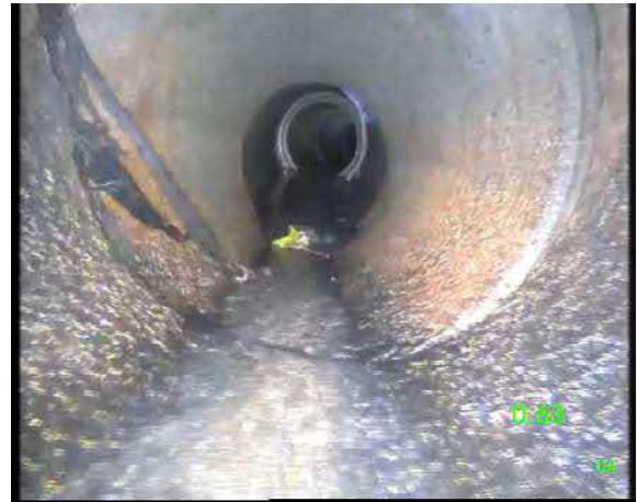
SMH1X_885ab768-8c54-405c-b348-cd1dca354b3f_20231019_215407_864.jpg, 00:00:20, 0.63 m Roots, fine at joint
