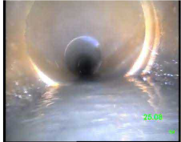
SMH1X_e10e47b0-9b97-4679-b11a-c3080e9dbed7_20231019_215813_462.jpg, 00:02:50, 25.08 m Joint displaced, medium
