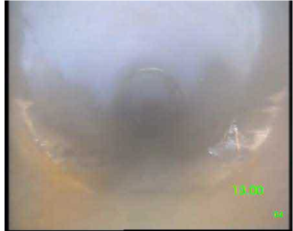
SMH1X_ea7c40a2-d2a6-43ca-905d-944eba992b6c_20231019_215615_174.jpg, 00:01:39, 13.05 m Roots, fine at joint
