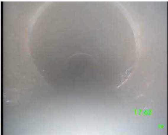
SMH1X_c29a90ee-f258-47c6-a05d-786affb5dbc7_20231019_215707_301.jpg, 00:02:06, 17.62 m Roots, fine at joint
