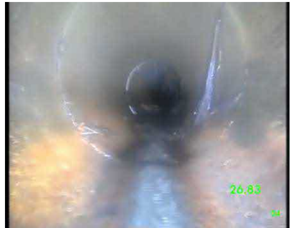
SMH1X_d305c559-ddb9-492d-b870-5d4fdb75086b_20231019_215832_566.jpg, 00:03:01, 26.87 m Roots, fine at joint
