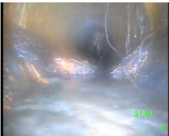
SMH1X_39e3fe2e-2cf7-4c61-a331-9cc1021f688a_20231019_215853_268.jpg, 00:03:07, 27.81 m Roots, mass at joint, 30% cross-sectional area loss
