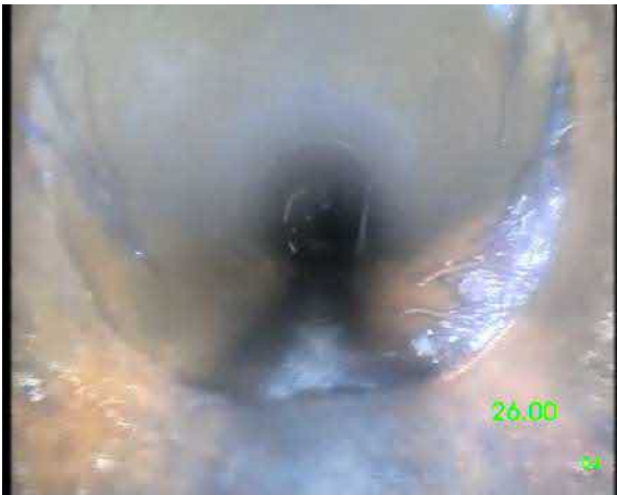
SMH1X_0ea55e5c-d473-4f04-abbb-7345b45689fe_20231019_215823_264.jpg, 00:02:56, 26.00 m Roots, fine at joint
