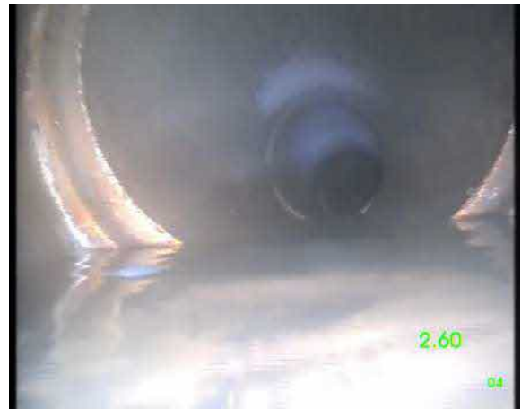
SMH1X_8a35c796-c733-40ce-ab8b-f39d3adb1ead_20231019_215447_341.jpg, 00:00:34, 2.60 m Joint displaced, medium
