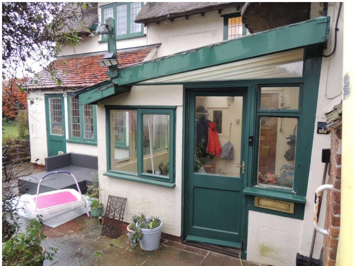
Photo 1: Western elevation. The proposal is for a single-storey extension in this area
