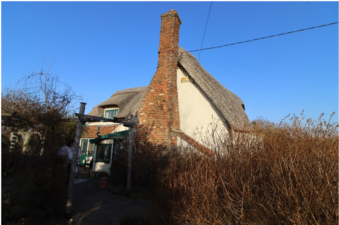
Figure 6. Chimney on West elevation to have repointing repair work using lime mortar.
