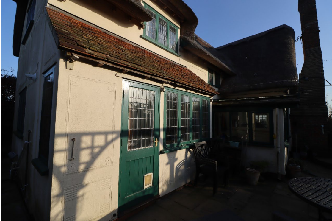
Figure 5. View of East elevation of the rear C20th extension and bay that is to be extended. C20th porch to be demolished is visible on the right.
