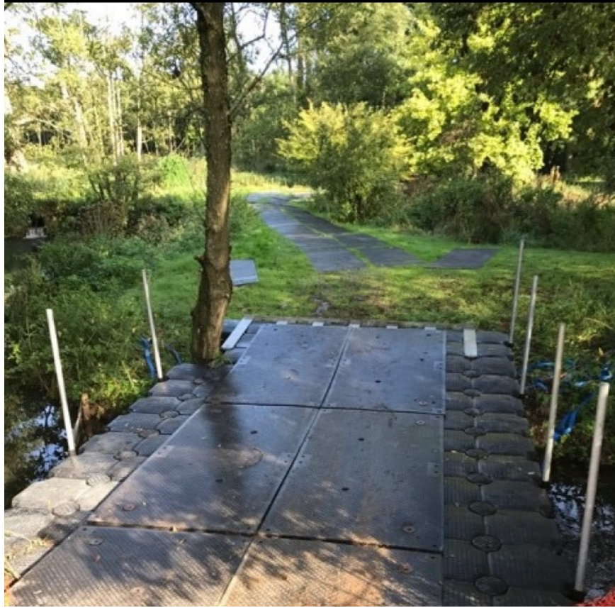
Fig. 2 Ground Guards – MultiMatts Euro Trak is ideal for the ground protection required here.
