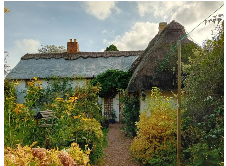
Figure 24 Rear of building, note tarp, west elevation, WHC
