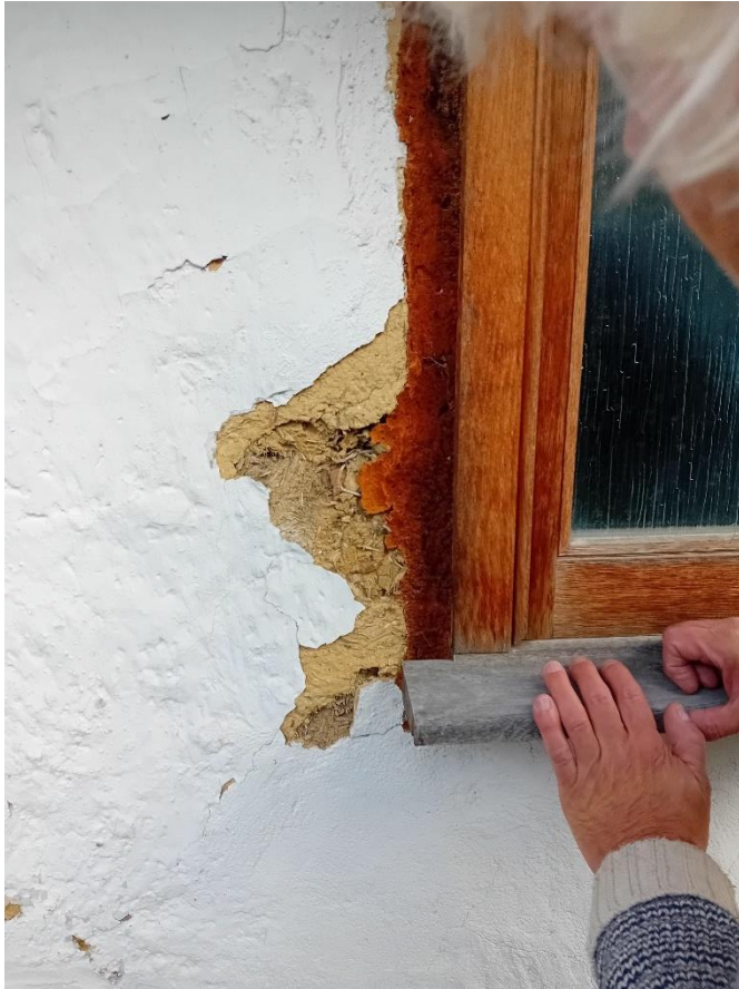
Figure 35 Detail of failed render and substrate, WHC
