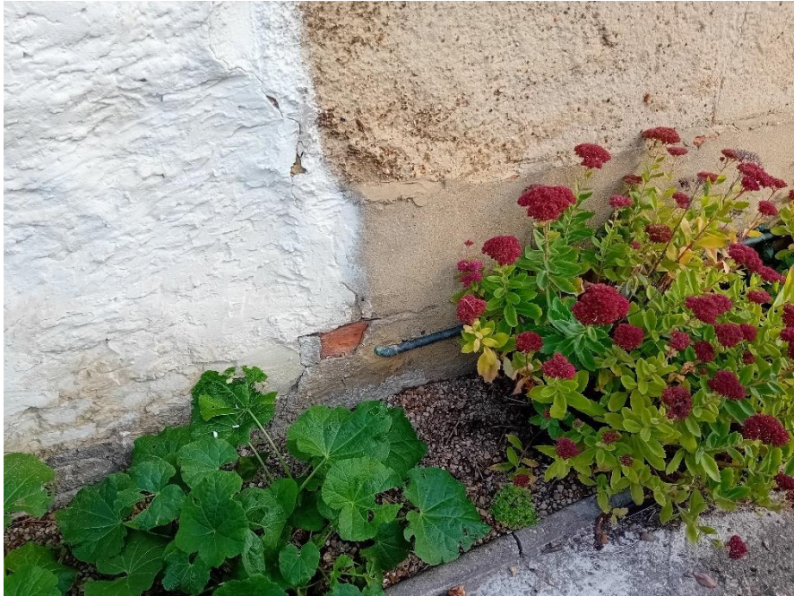
Figure 37 Base of render at ground, WHC
