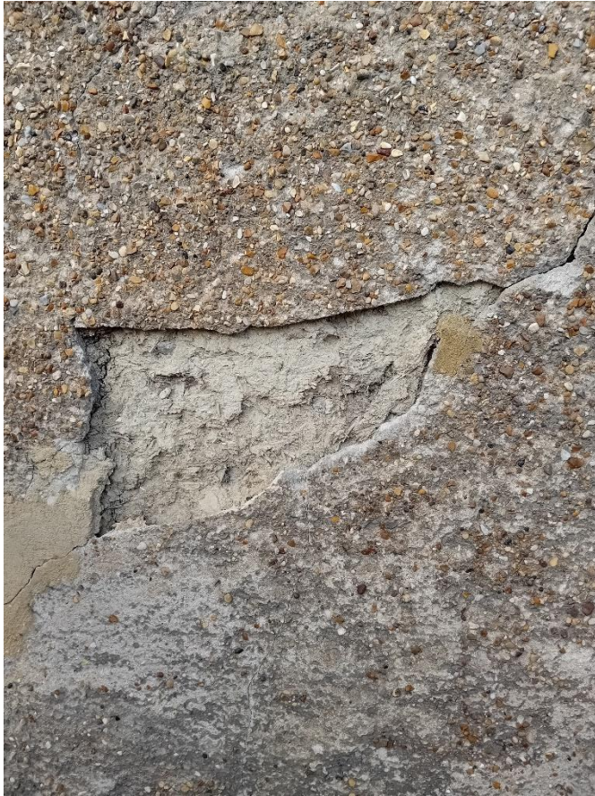
Figure 33 Detail of failed render and substrate, WHC
