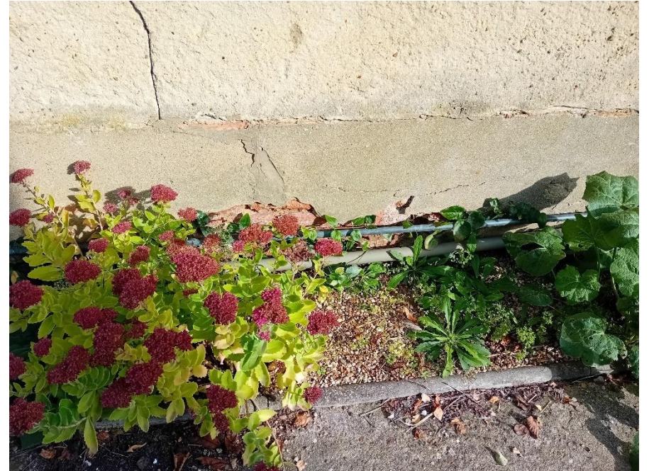
Figure 38 Base of render at ground, WHC
