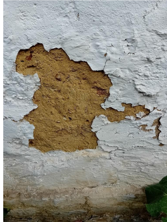
Figure 34 Detail of failed finish and substrate, WHC
