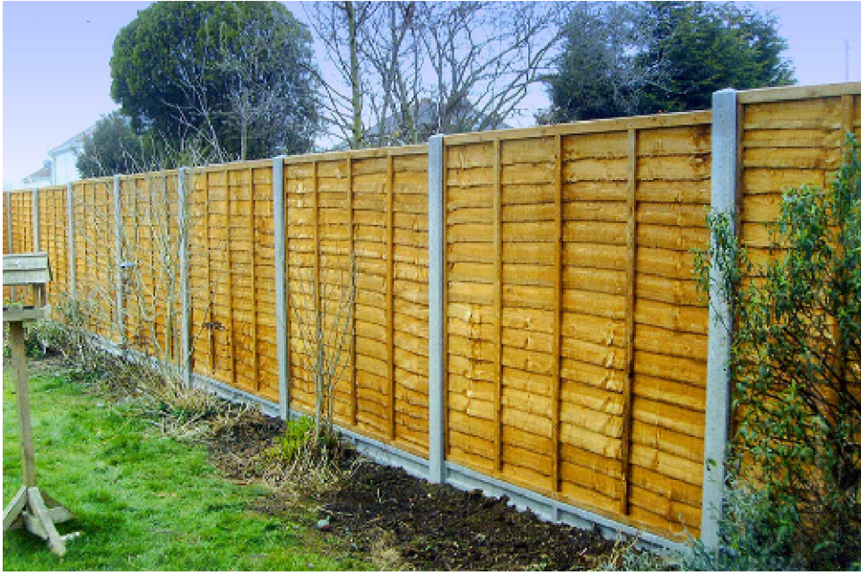
1.8m high panel fence with concrete posts & gravel boards to match existing
