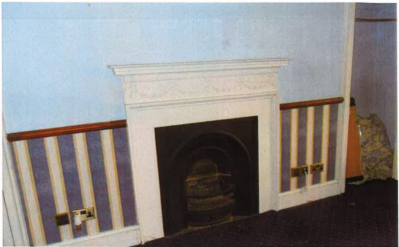
Appendix 4.27: 19th century fireplace located within the rear room at second floor level
