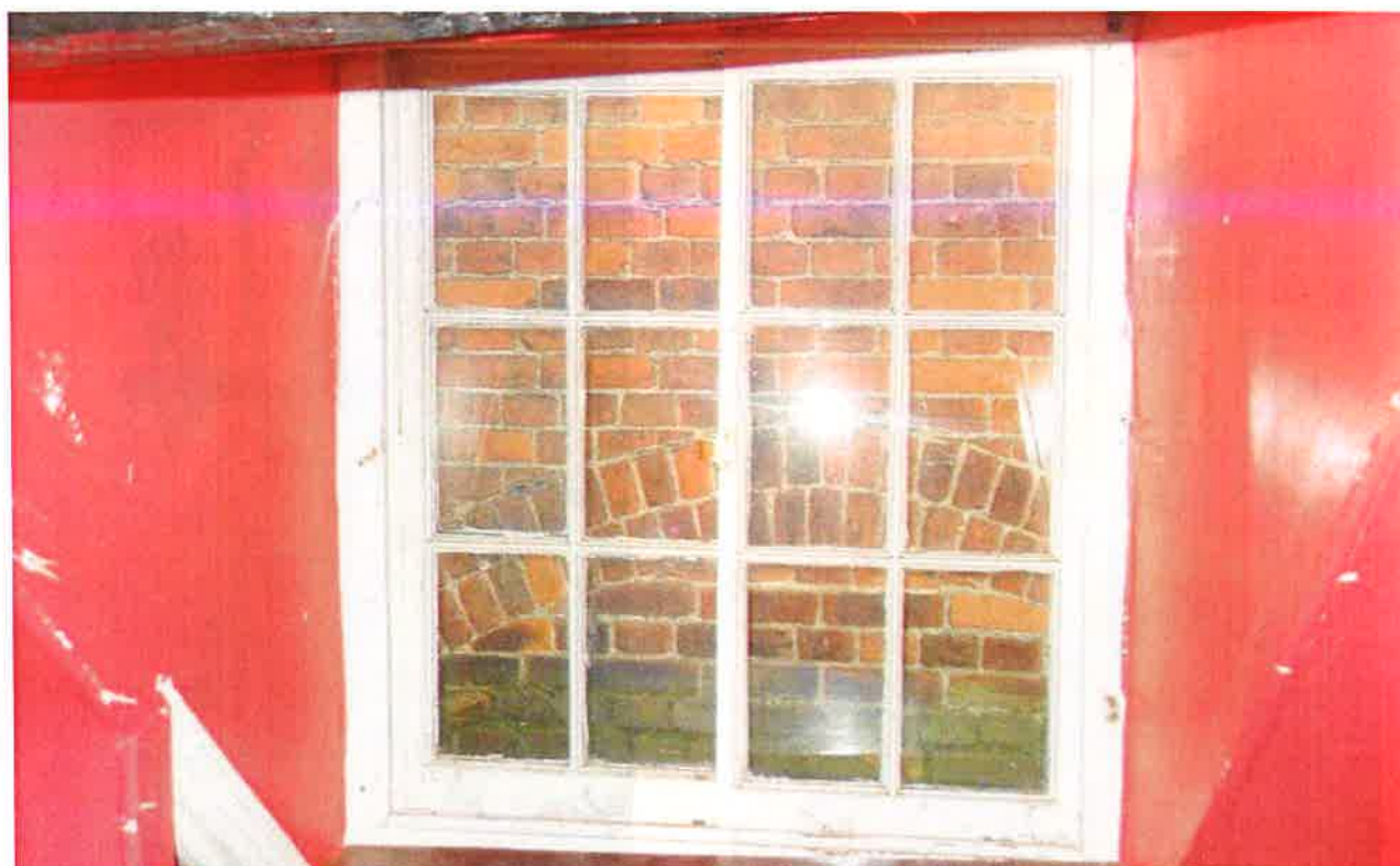
Appendix 4.26: Second floor window proposed for conversion to a doorway with corridor leading to the room beyond where a past opening has previously been located
