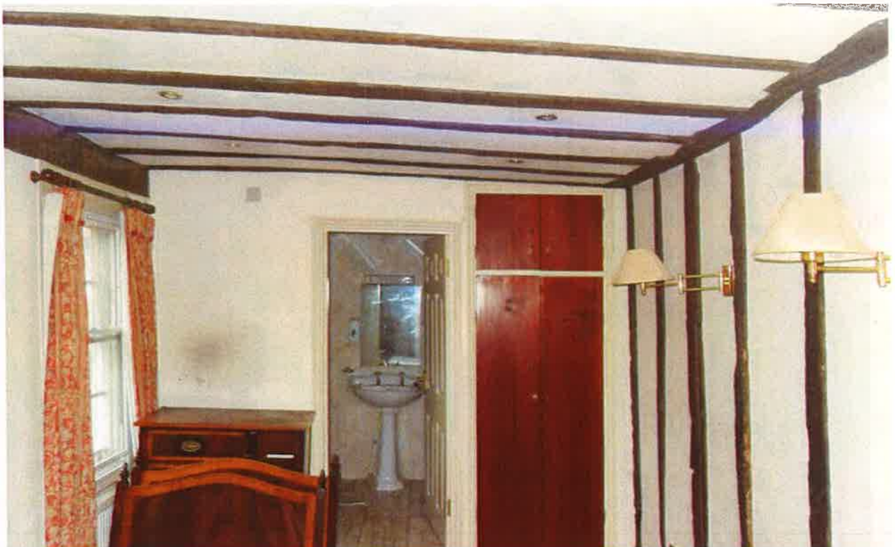
Appendix 4.24: Second floor front room with exposed timber framing and later partitions
