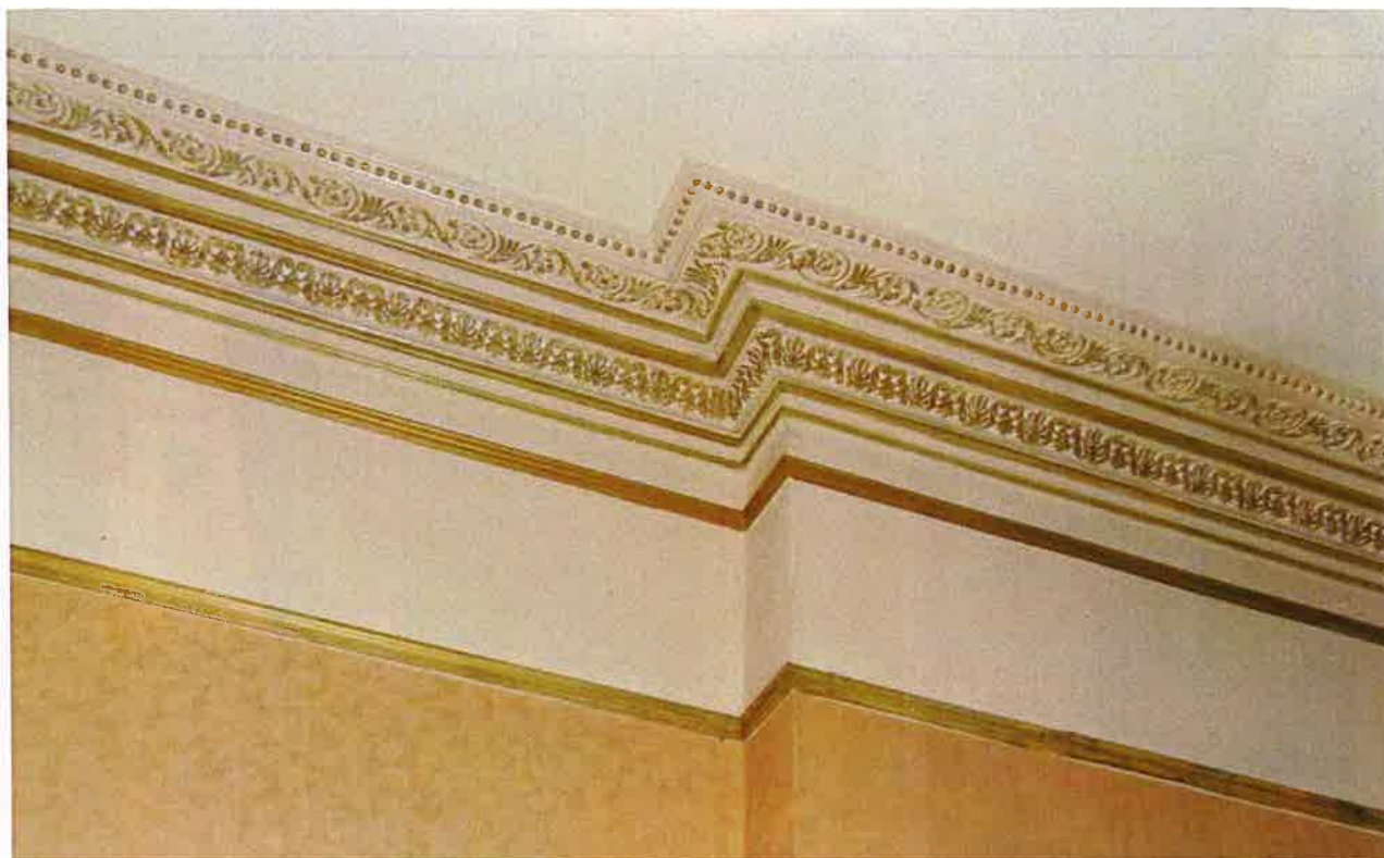
Appendix 4.35: Cornice detailing within the late 19th century room at ground floor
