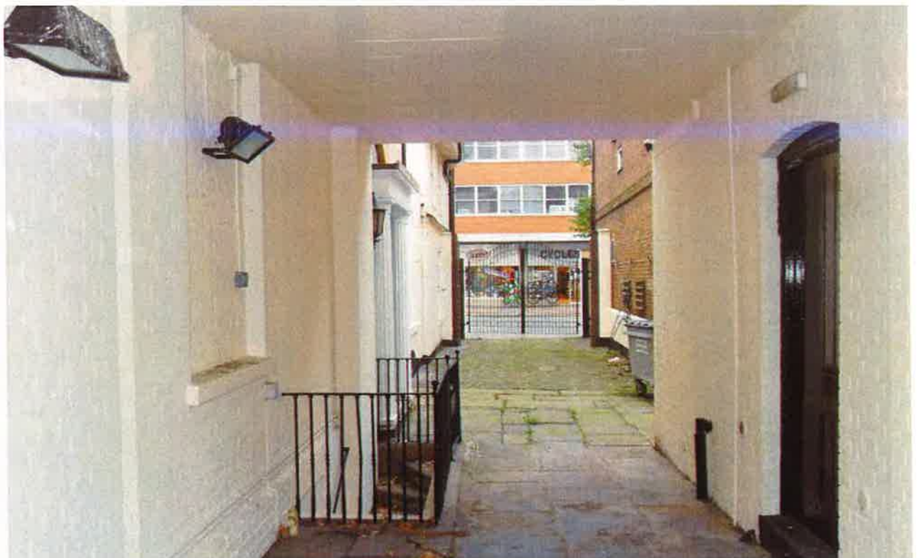
Appendix 4.6: Underpass of flying freehold with boiler room to the right hand side and main body of the Stone Court Hotel to the left
