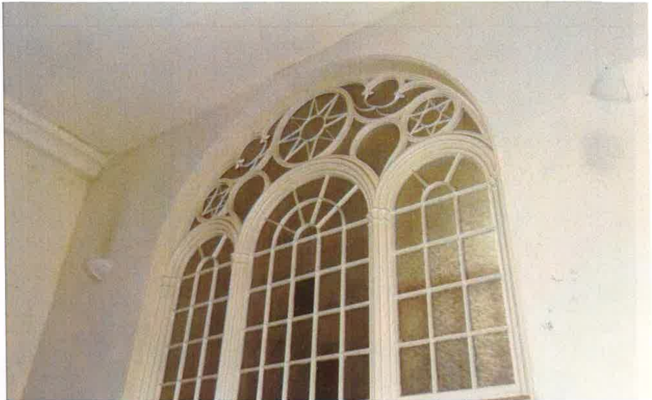
Appendix 4.14: Large arched window providing light at landing level within the staircase
