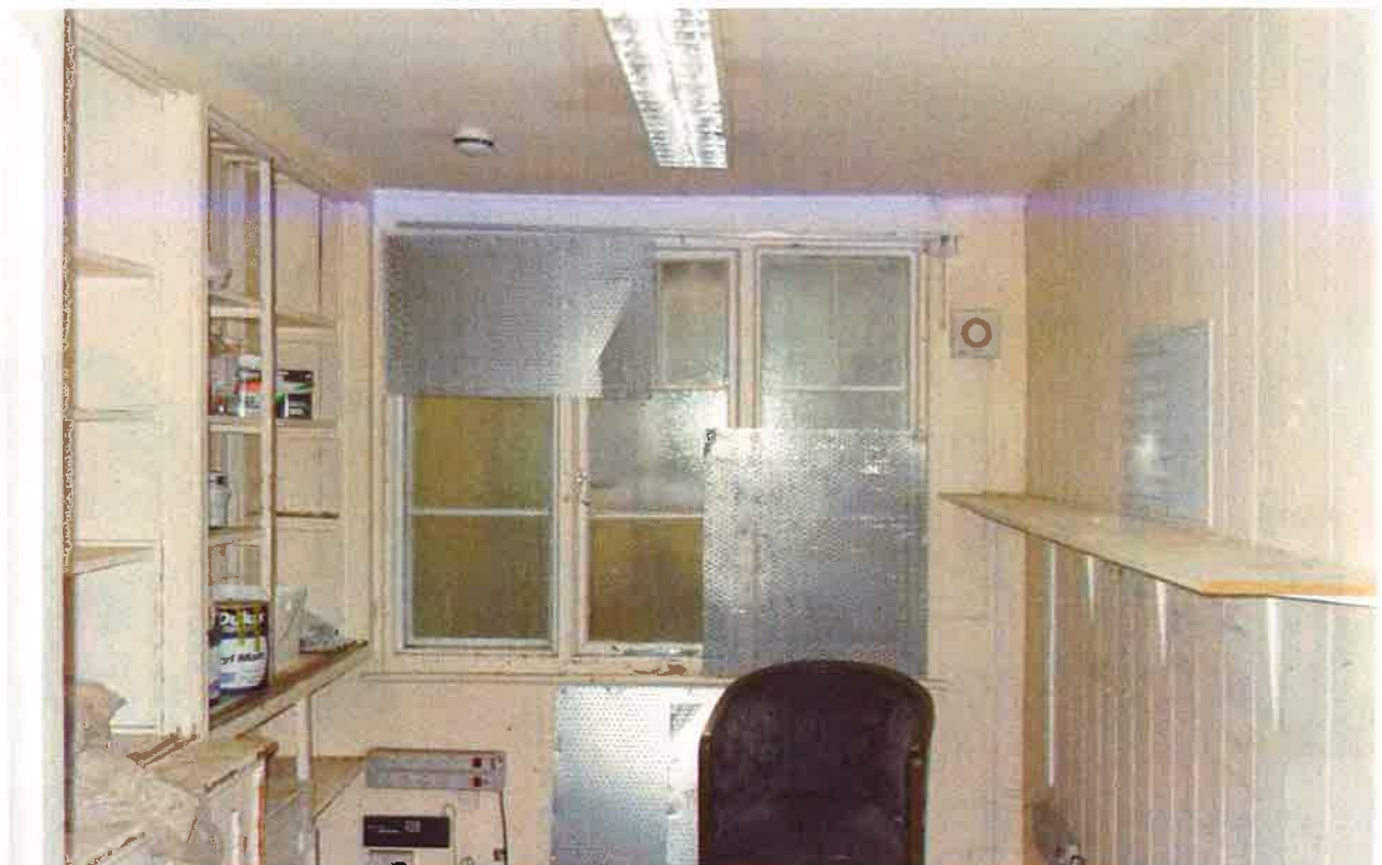
Appendix 4.38: Housekeepers room dating to the late 19th century proposed for removal to facilitate the opening of the courtyard
