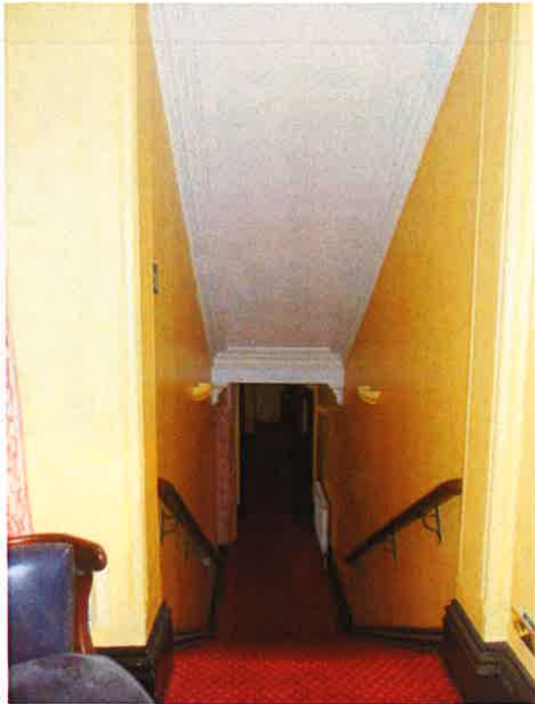
Appendix 4.39: Late 19th century corridor to be removed to open the courtyard
