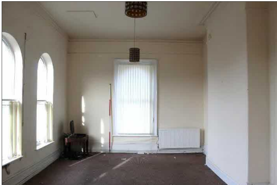
Plate 36 (shot 86): General view of room 1.1 with blocked fireplace to the right and later skirting board. Looking northwest, 2m scale
