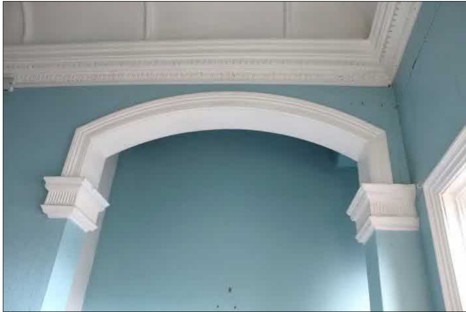
Plate 35 (shot 67): Close up of moulded architectural features with egg and dart motif and dentil above on the cornice and reeding on the corbels. Looking northwest
