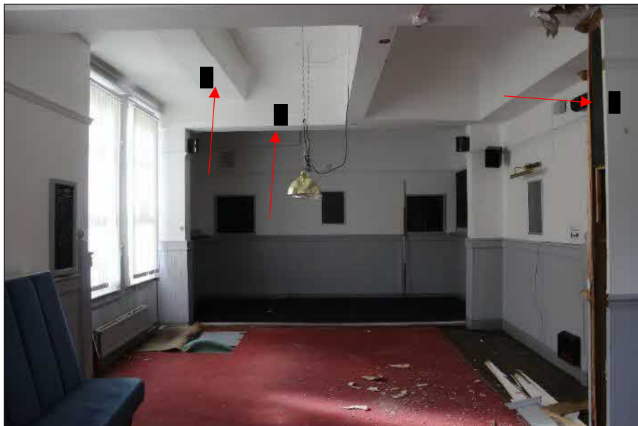
Plate 28 (shot 130): General view of Lounge 3. Arrows point to locations of removed walls Looking southwest, 2m scale
