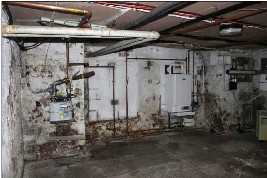
Plate 9 (shot 162): General view of southwest cell (A0.1), showing two blocked cellar windows on the southwest wall. Looking west-southwest
