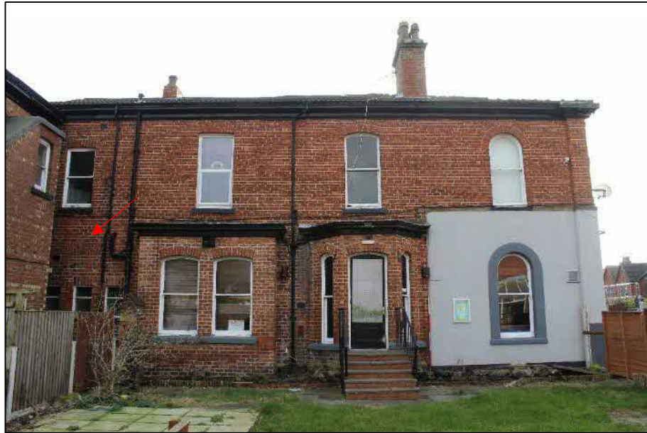
Plate 7 (shot 23): Close up of northwest elevation of the main hotel structure (A). Arrow points to blocked opening. Looking southeast, 2m scale
