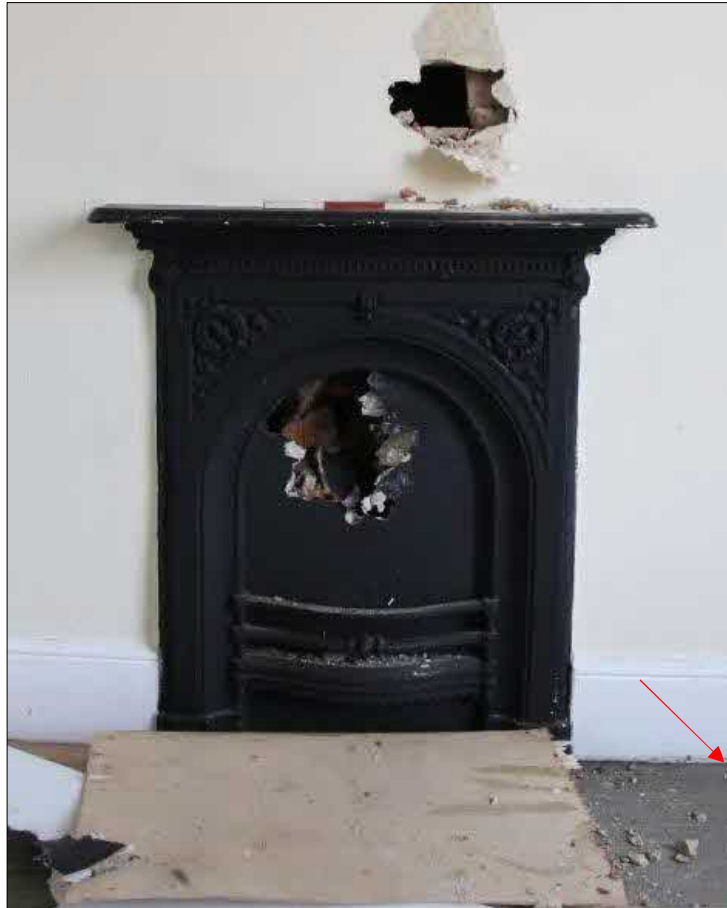
Plate 42 (shot 79): Close up of boarded up fireplace in 1.5. Arrow points to edge of hearth Looking southwest, 0.3m scale
