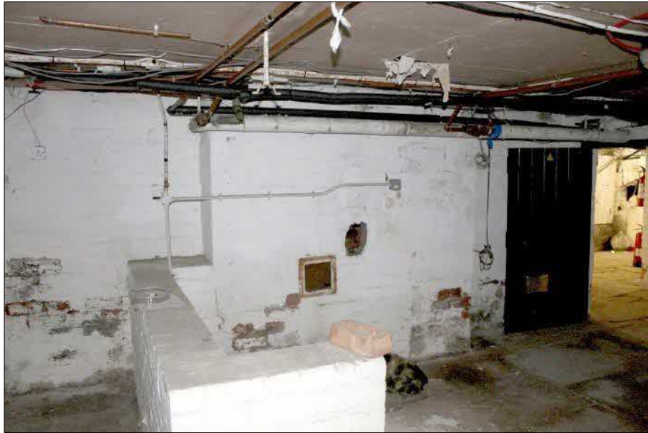
Plate 10 (shot 164): Bricked up fireplace on the northeast wall in A0.1. Looking east-northeast
