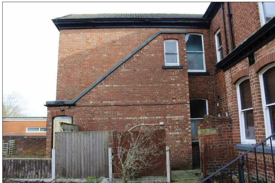
Plate 8 (shot 34): View of added staircase to the southeast wall of the northeast wing. Looking northeast
