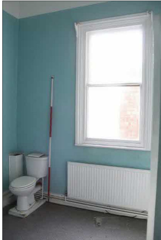
Plate 45 (55): General view of bathroom 1.7, in the northwest wing. Looking west-northwest, 2m scale
