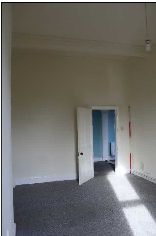
Plate 39 (shot 69): Bedroom 1.4 showing an extra beam in the ceiling. Looking northwest, 2m scale
