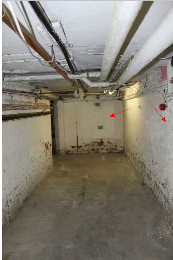
Plate 14 (shot 150): View of cellar corridor, arrows point to blocked openings. Looking northeast, 1m scale
