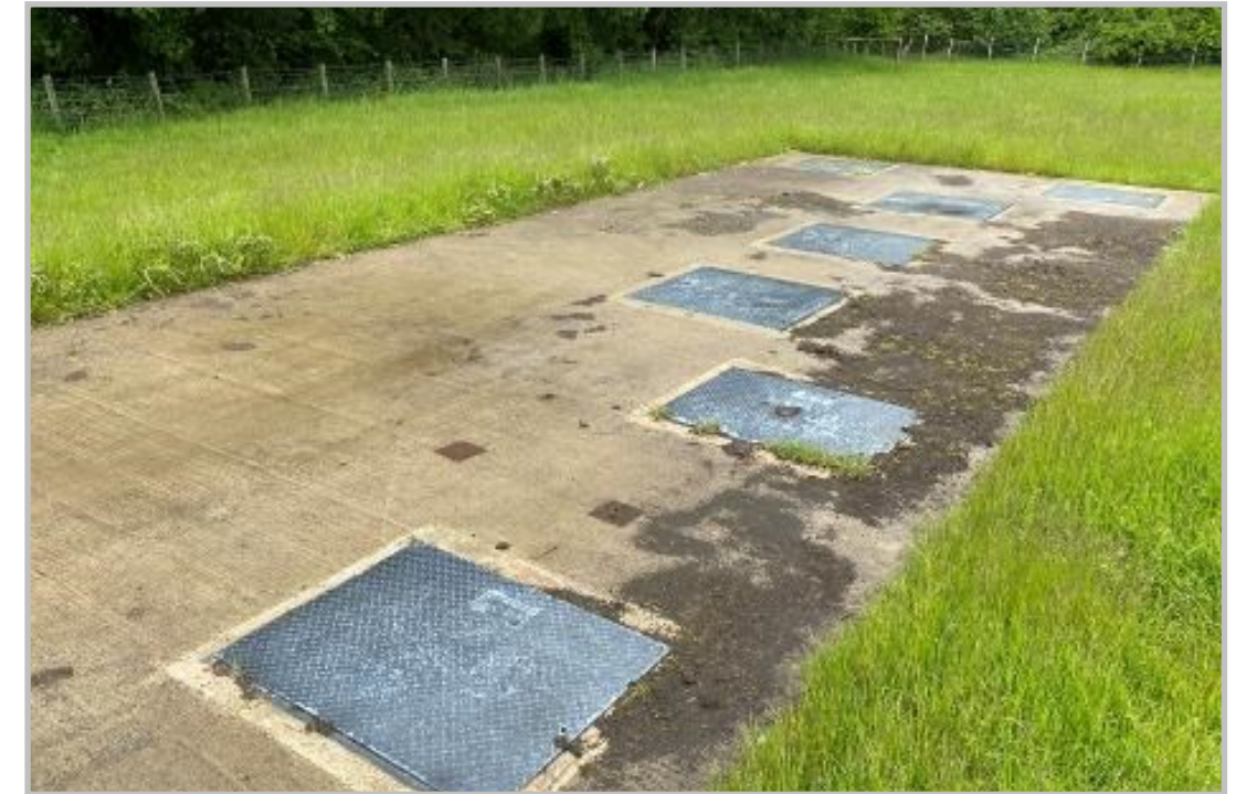
Existing utility facility within the site
