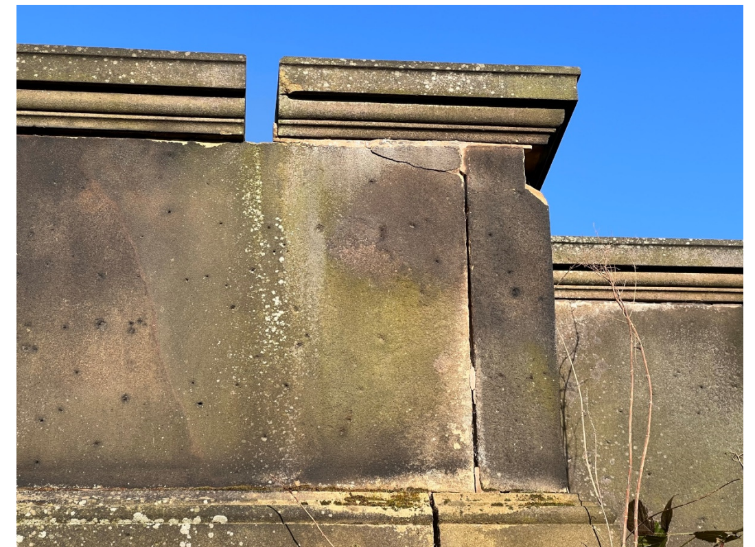
Figure 9 – Defects at staircase return showing cracking and movement.
