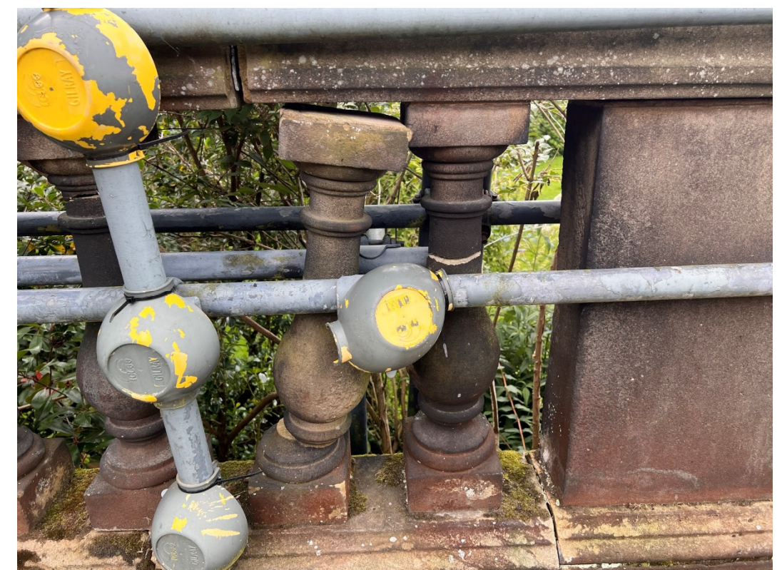
Figure 12 – Loose and fractured balusters with scaffolding supports.
