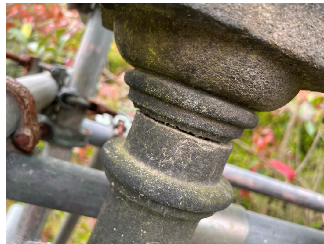
Figure 3 – Typical Cracking to Balusters
