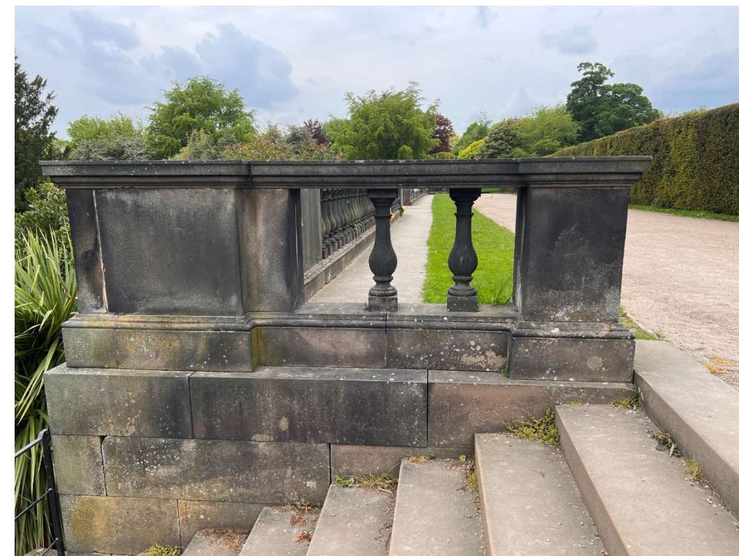
Figure 10 – Staircase showing missing balusters.
