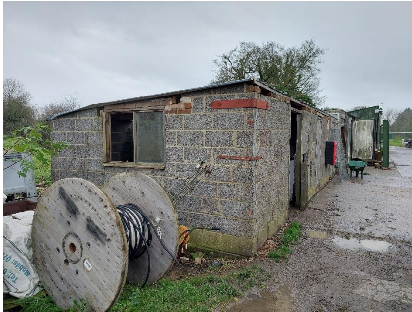
Figure 2 - Dilapidated buildings, to be removed.
