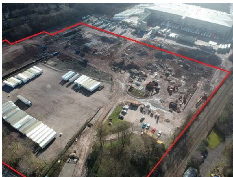
Figure 1 – Aerial image of the site dated 7 th March 2023, looking south east. Demolition works in progress. Site boundary shown in red.
