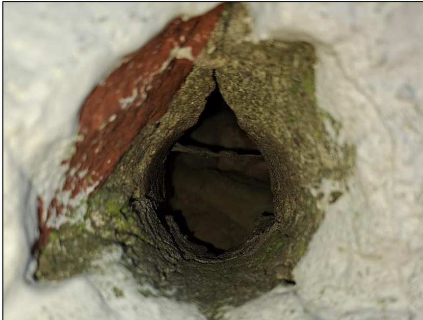
Photograph 4 showing the hole in the brickwork
