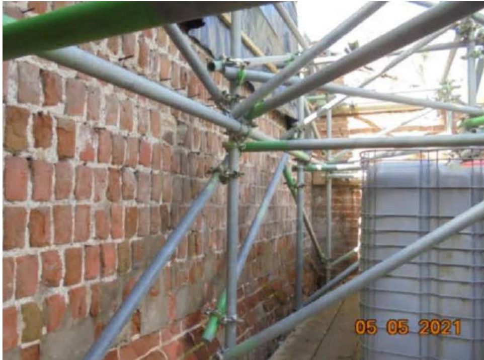
Image above: structural supports within Clay Lane Cottage on 5 May 2021
