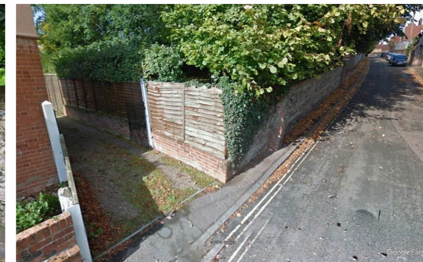
VIEW OF RETURN PRIOR TO COLLAPSE © GOOGLE EARTH
