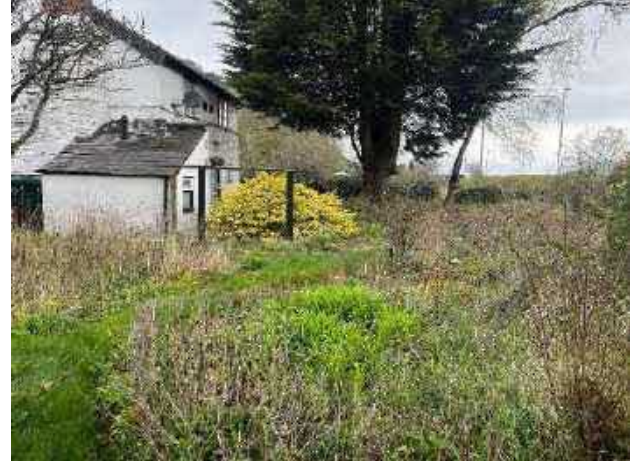
P16: View of the eastern wall of the cottage and land immediately behind facing north-east
