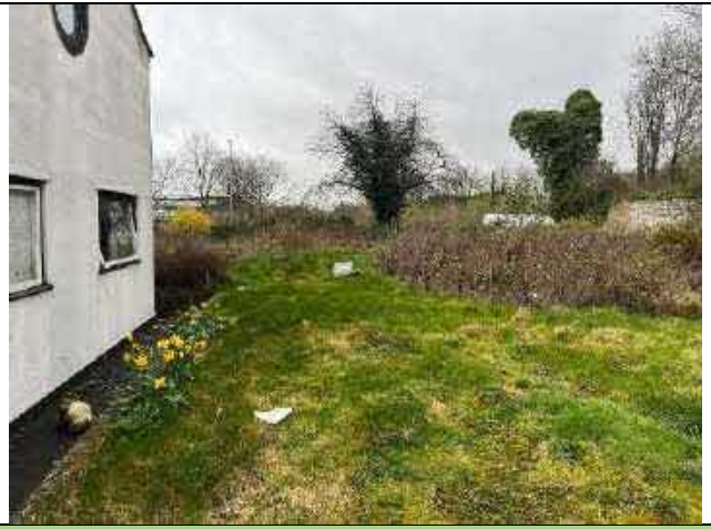
P8: View of the western wall of the cottage and end of the driveway facing south-west
