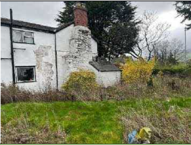
P13: A view of the southern wall of the cottage facing north
