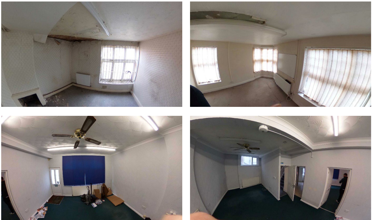
Figure 2. Internal images to show current poor condition
