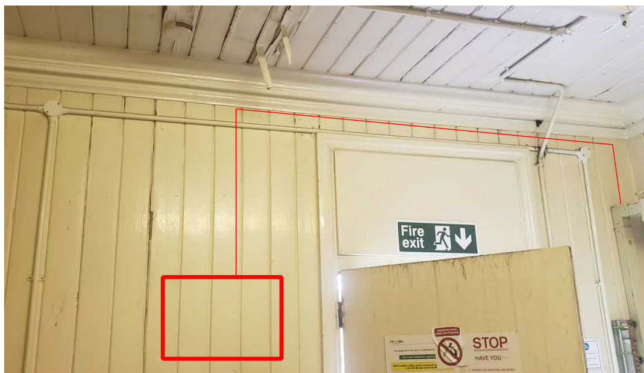
Figure 72: Proposed Platform 1&2 Help Point Equipment, Position of Fused spur and PSU with conduit route
