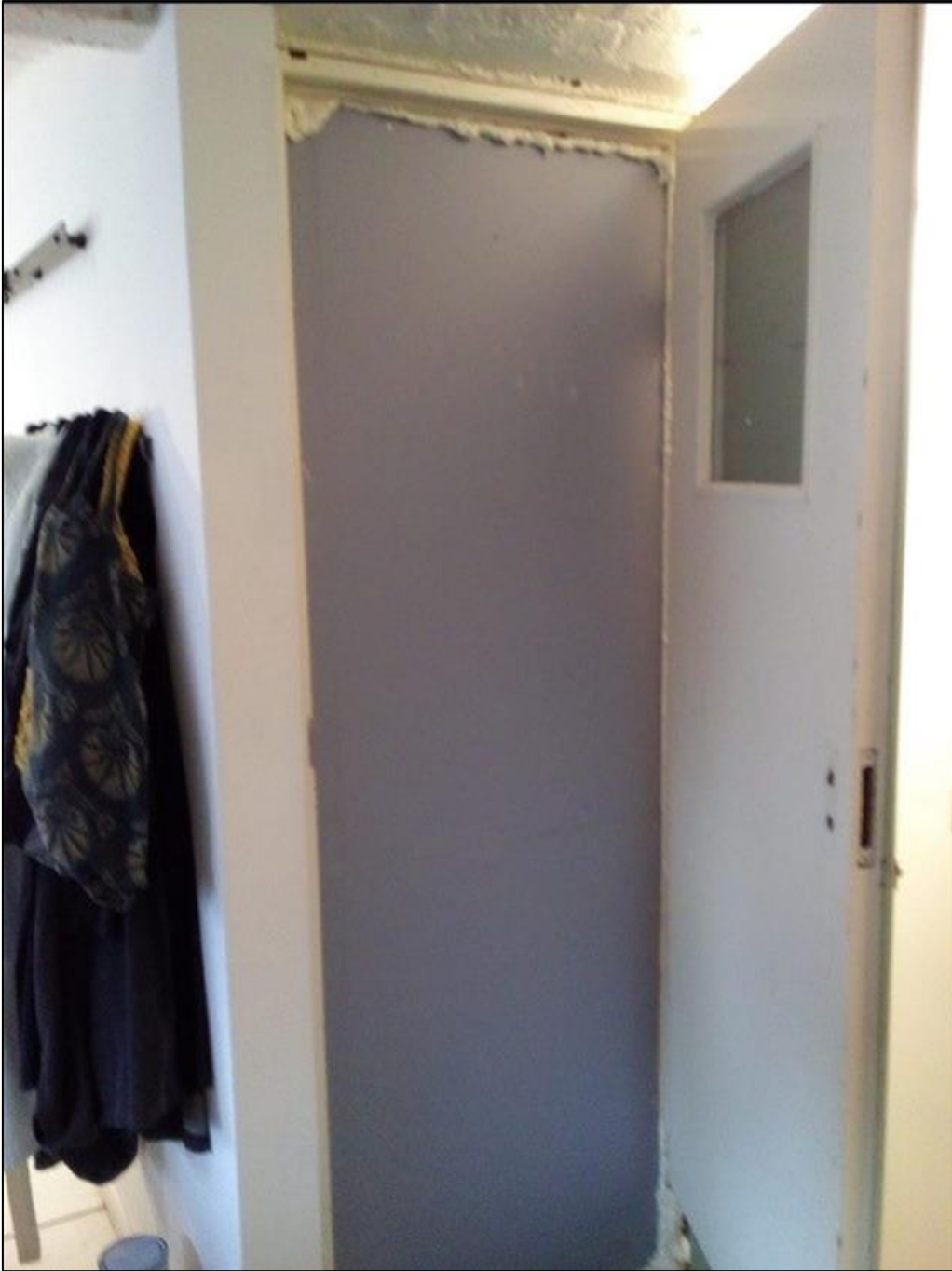
Blocked staircase to the rear of 23B Cambridge Grove
