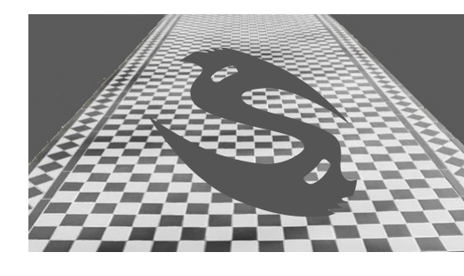
15 No. 131 - Central recessed entrance finished in porcelain tiles with inset dark grey/black company logo.
