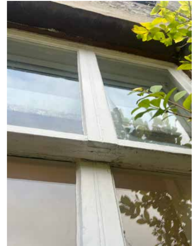
2. Separating joints and rotting edges
