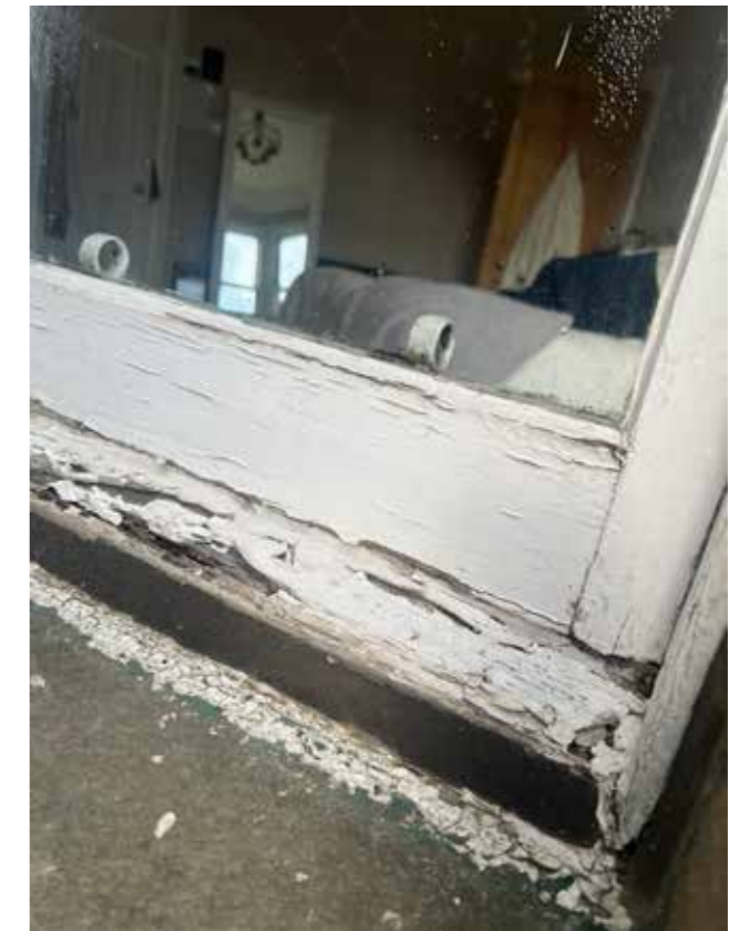
4. Rotting sill and open joints
