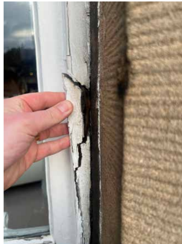
3. Rotted through linings
