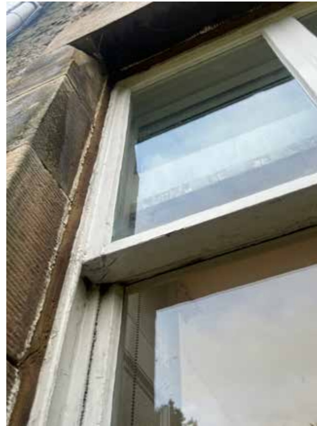
1. Split end grain and rotting edges
