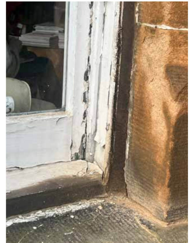
4. Rotting sash, flaking paint and open joints
