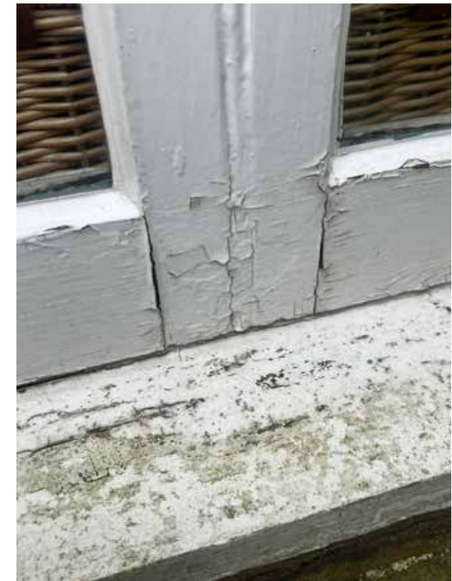
4. Rotting sill and open joints
