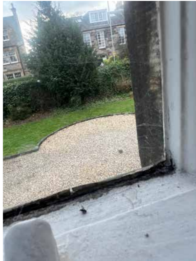
1. Rotting seal around glass
