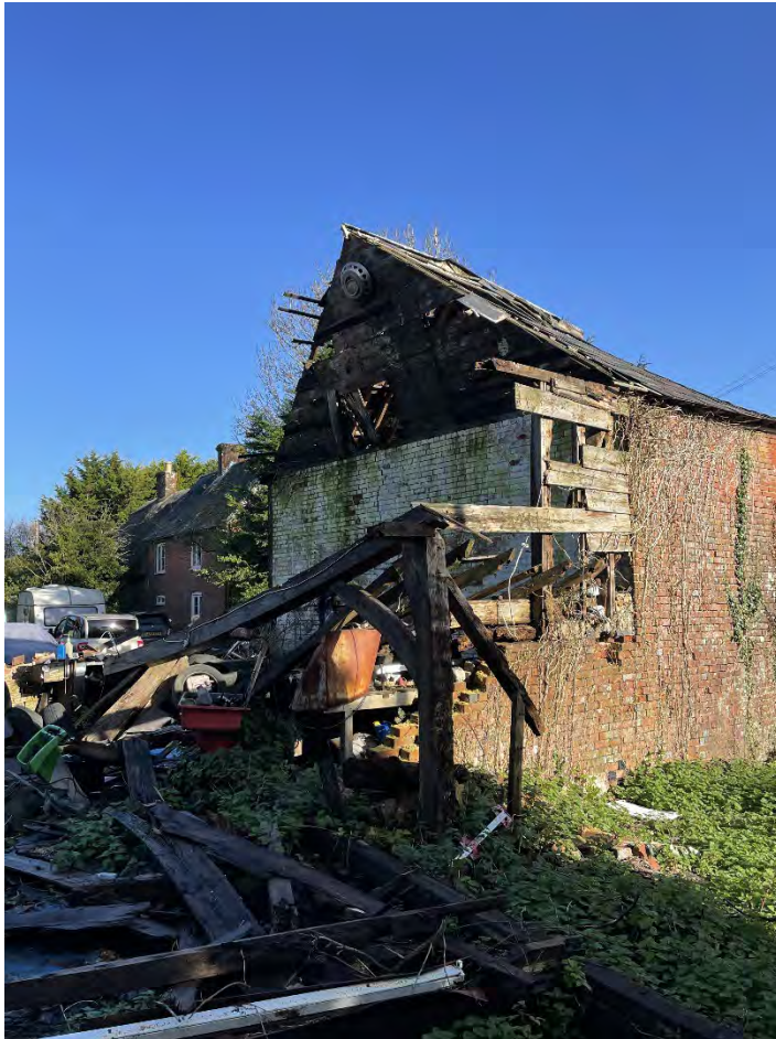
Plate 35: Western part of Building B that has entirely collapsed.
