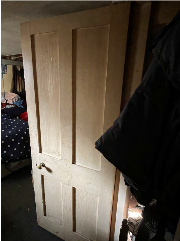
Plate 26: Old Farmhouse, example of four-panel door with keyplate and lock case on the ground floor of the historic core.
