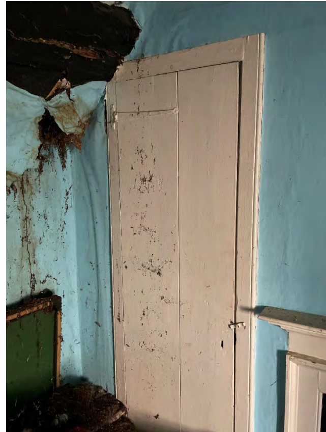
Plate 25: Old Farmhouse, example of plank door with round end strap hinge on the first floor of the historic core.
