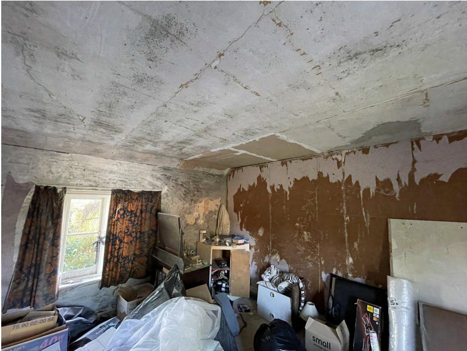
Plate 22: General view of the southernmost first-floor room with evidence of ceiling collapse and repair with plasterboard.
