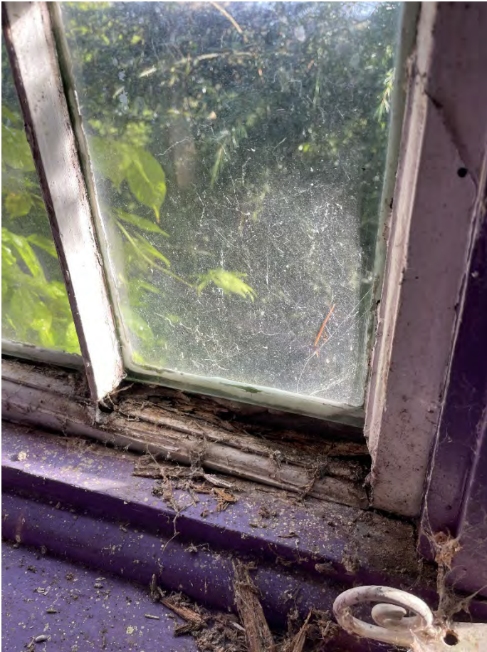
Plate 24: Detail of Plate 23 showing rotten timber.
