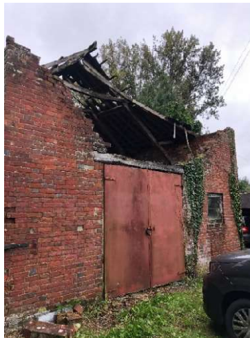
Fig 9 & 10: Views of the existing dilapidated outbuilding (Building 4)
