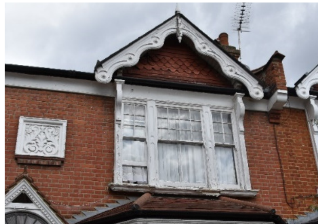
Windows and cills have deteriorated with lack of maintenance
