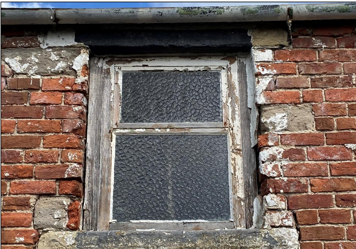
Plate 12: Window on the south facing aspect of the rear barn had gaps between the frame and the brick walls, offering PRFs and access into the internal spaces.
