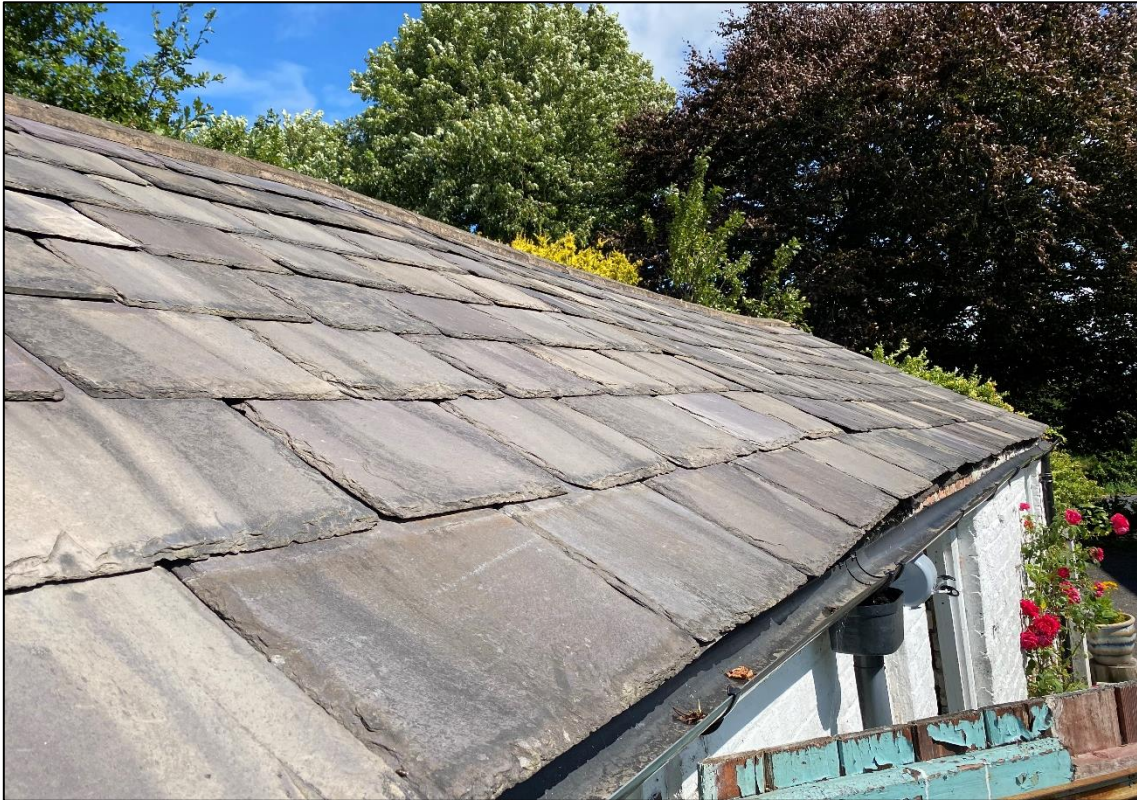
Plate 7: Slate tiles and ridge tiles on the outbuilding were generally tight fitting and in good condition.
