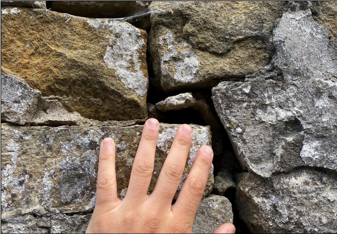
Plate 11: Large gaps were inspected with an endoscope and no evidence of bat presence or activity were found.
