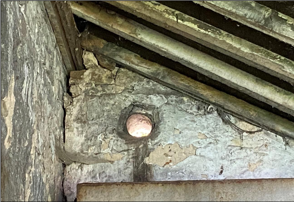
Plate 21: Gaps and cracks offering PRFs were identified in the garage.
