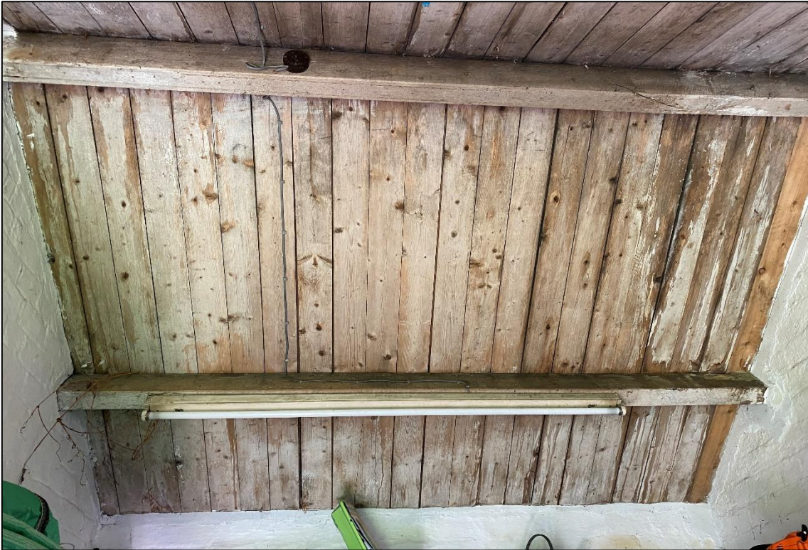
Plate 19: The outbuilding had timber boarding beneath tiles making the underside of the roof un-observable.
