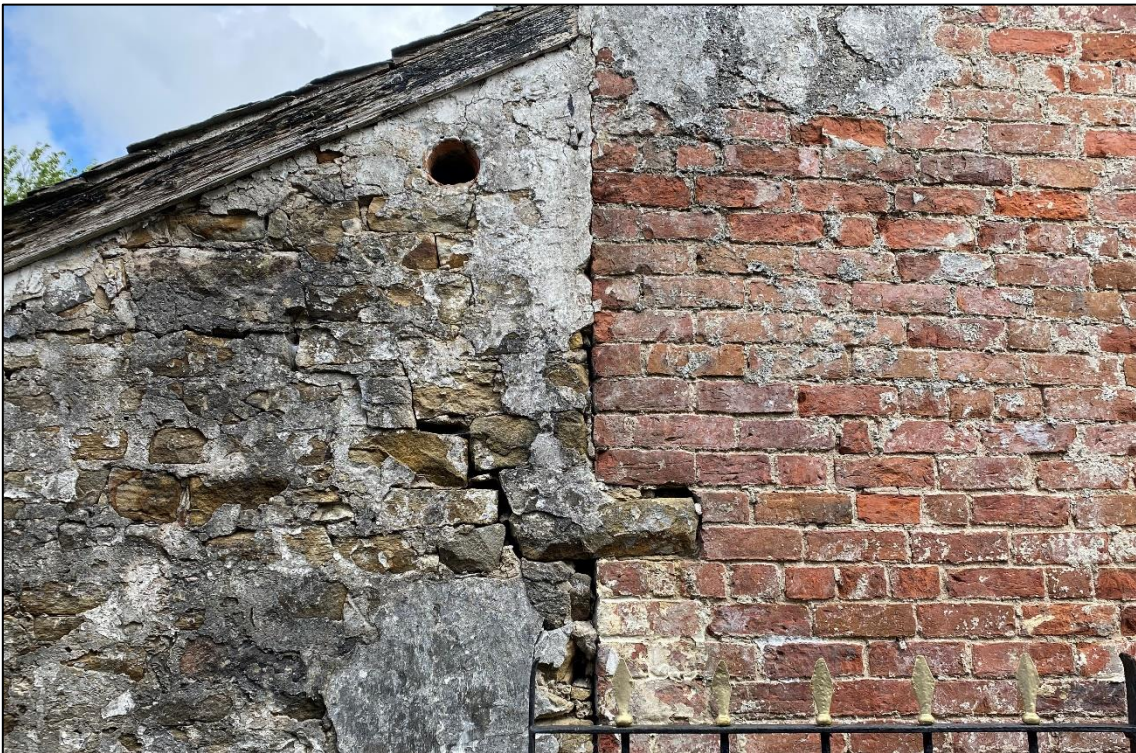
Plate 10: Large gaps and cracks in the brickwork of the main building offer PRFs.
