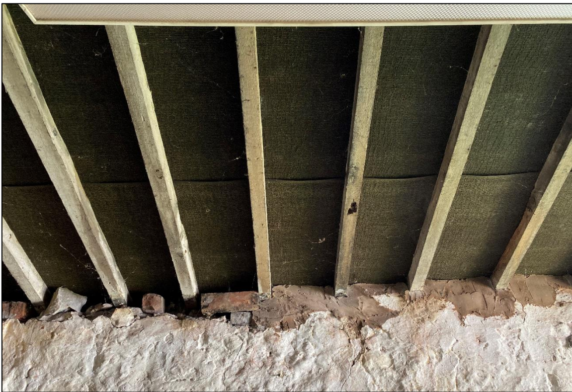
Plate 18: Timbers and membranes in the garage were exposed and intact. No bats present.
