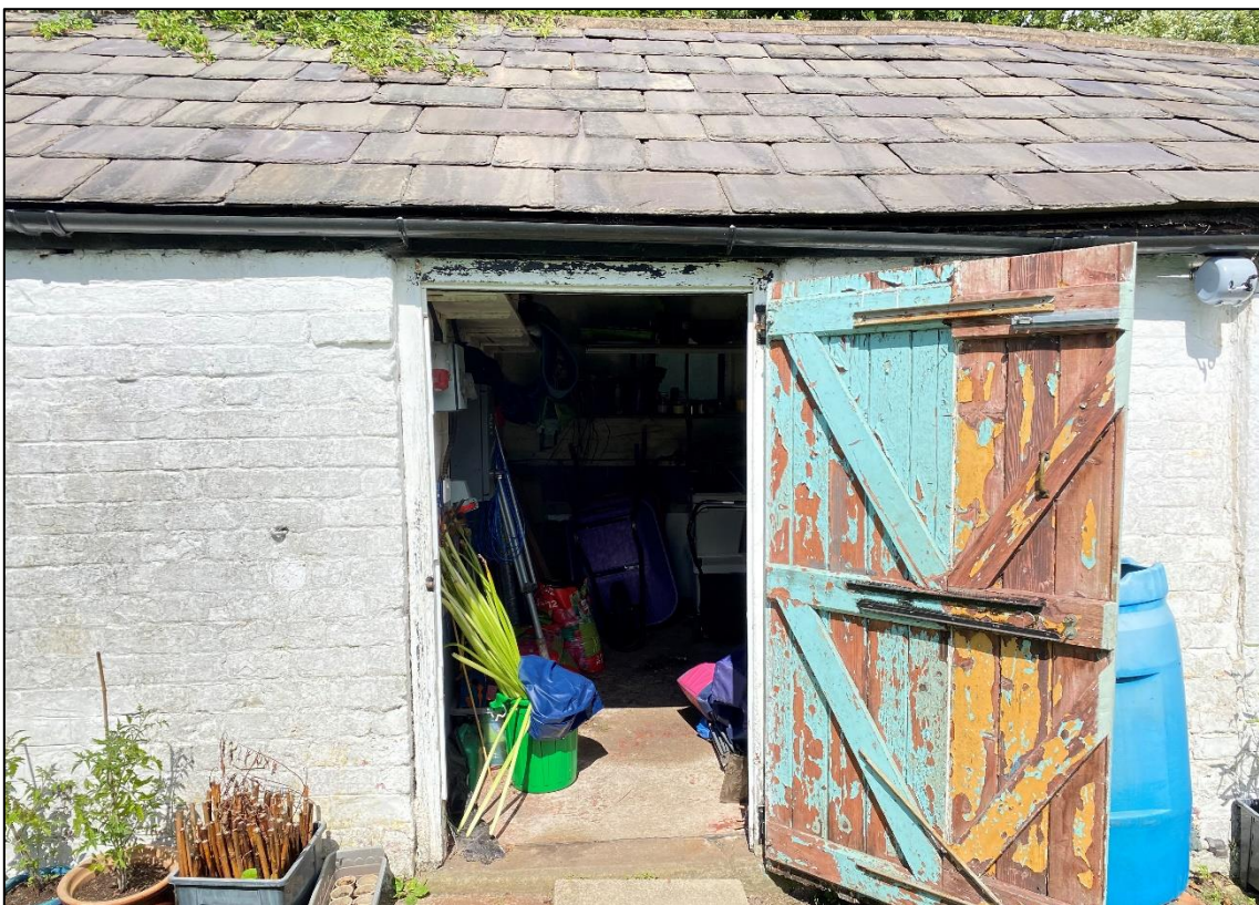
Plate 16: The outbuilding was divided into three sections which were open spaces with no ceilings.
