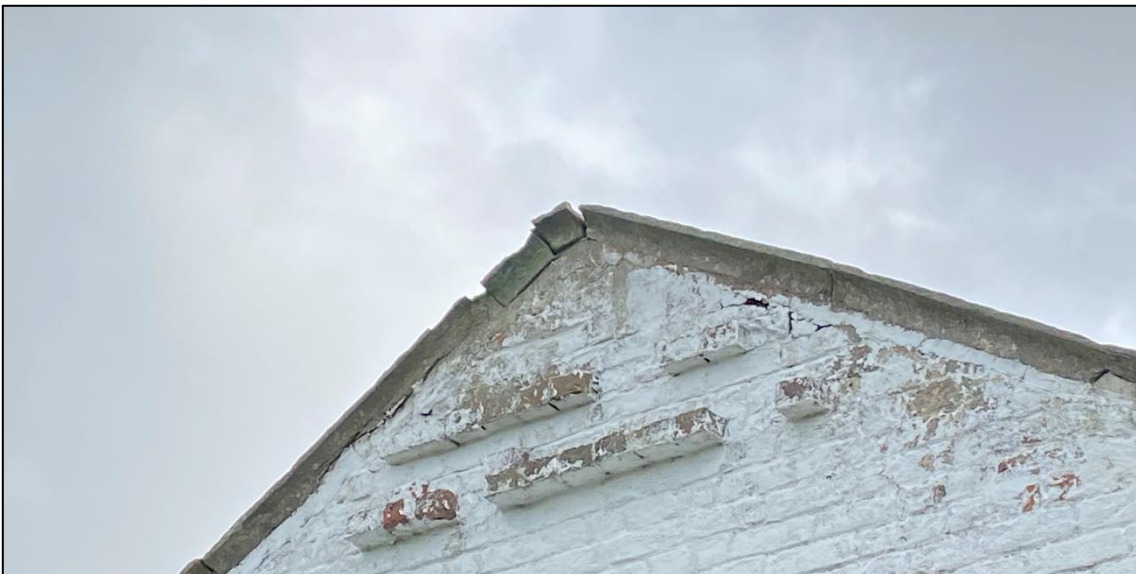
Plate 4: Cracks in the mortar beneath and between coping stones offers gaps for roosting.
