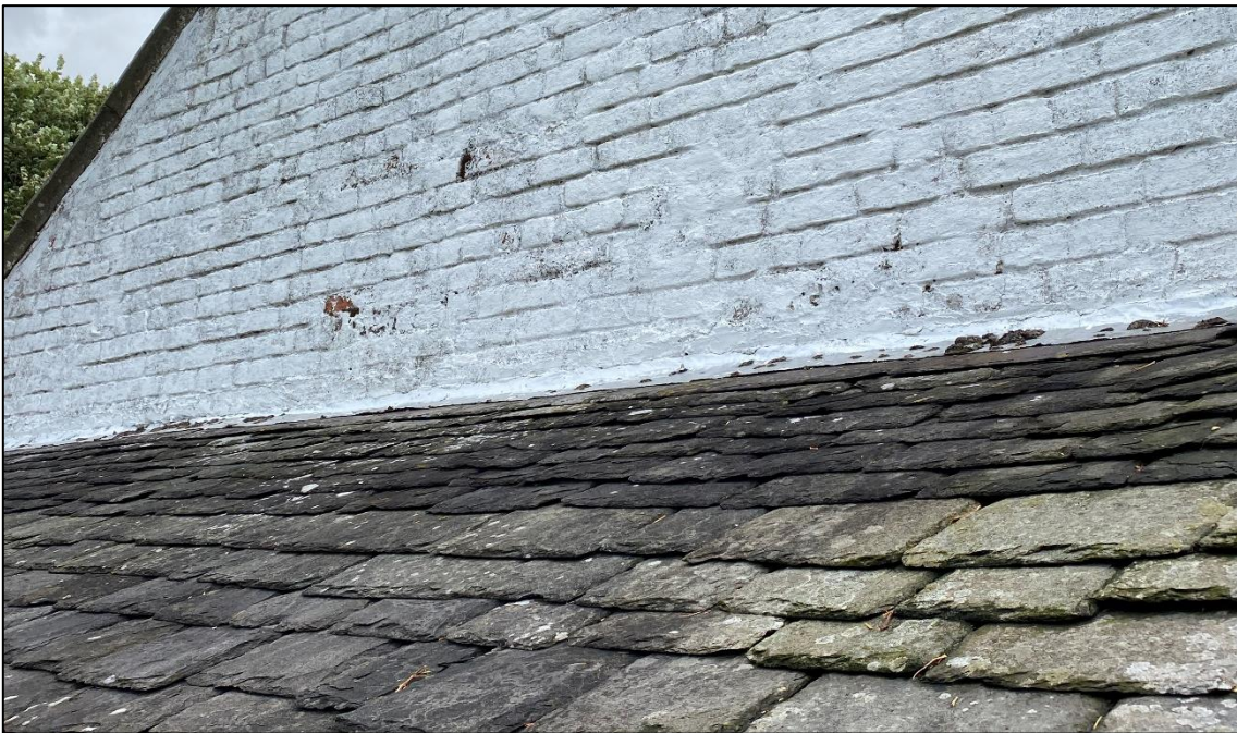
Plate 6: Flashing between the lean-to garage roof and gable of the barn was well sealed.
