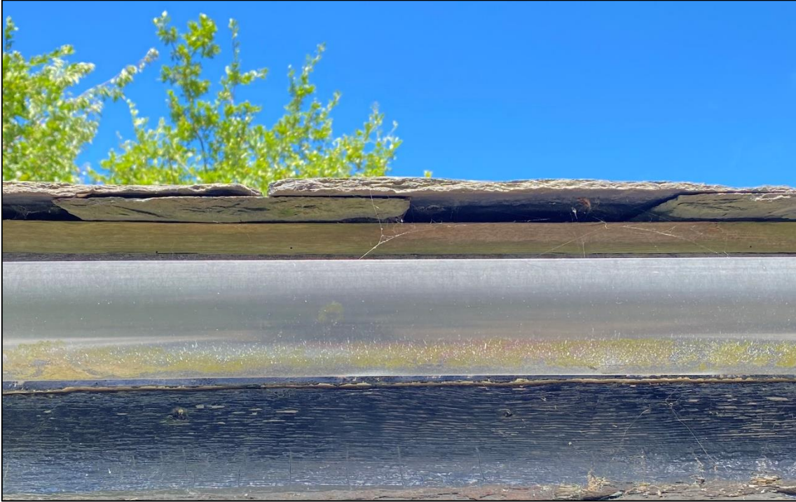
Plate 9: Fascia boards had guttering attached and were generally tight fitting. Gaps under slates along the roof edge offer PRFs and access for bats.
