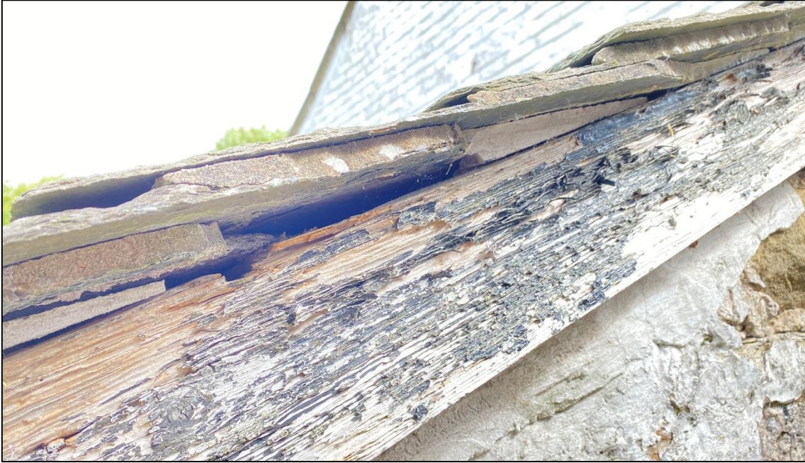
Plate 5: Gaps in the verges of the lean-to garage roof, offering PRFs.
