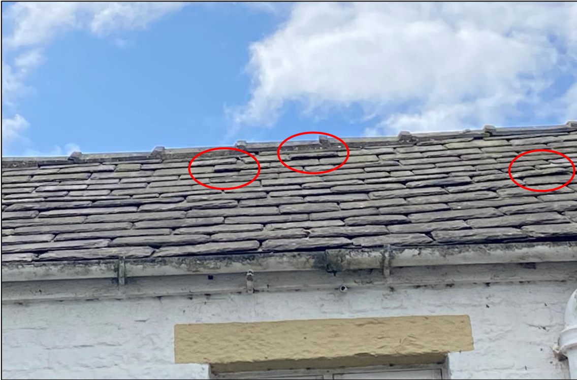
Plate 3: The pitched roof and ridges were generally in good condition but with lots of gaps beneath slate tiles offering PRFs.
