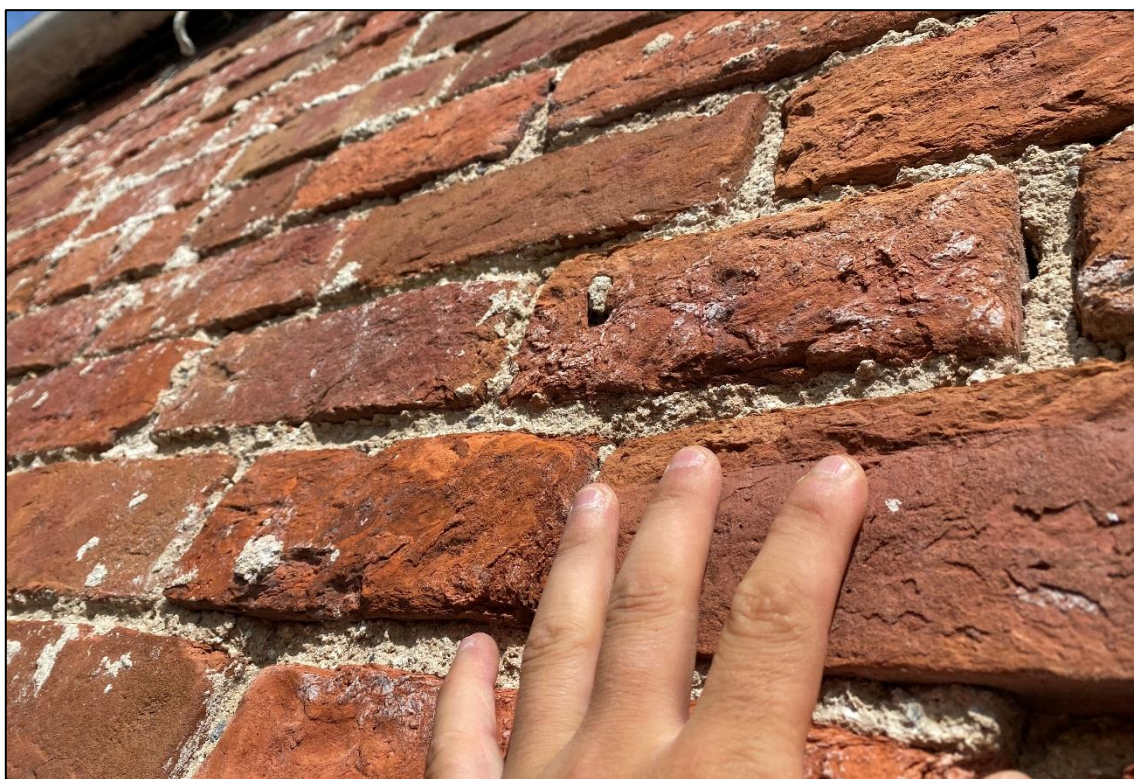
Plate 13: No evidence of bat activity was found on the external surfaces around the site.
