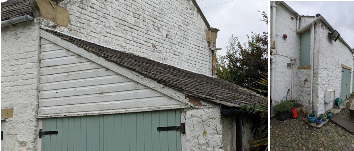
Failing fabric and plastic rainwater goods- proposed to be replaced and repaired, photographed Aug.2022
