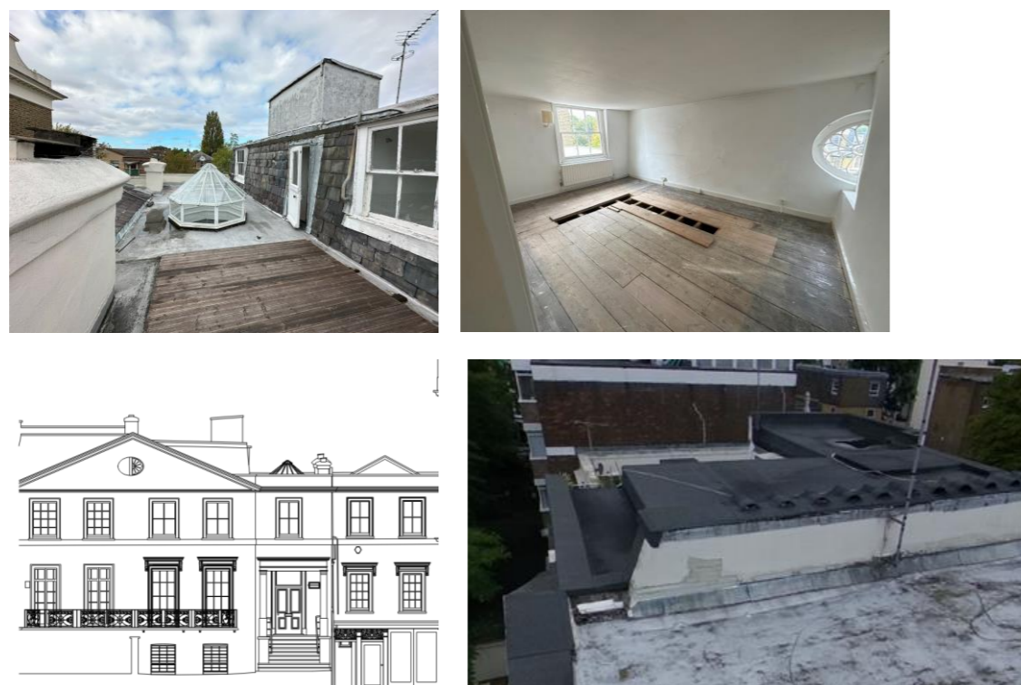
Figures 35-38: (clockwise from top left) Photograph of existing roof with incongruous water container; Internal photograph of the 2 nd floor show change in direction of the joists indicating later section of roof; Exact from the front elevation showing higher roof to no.20; Image of the stepped profile of the roof to no.20.
