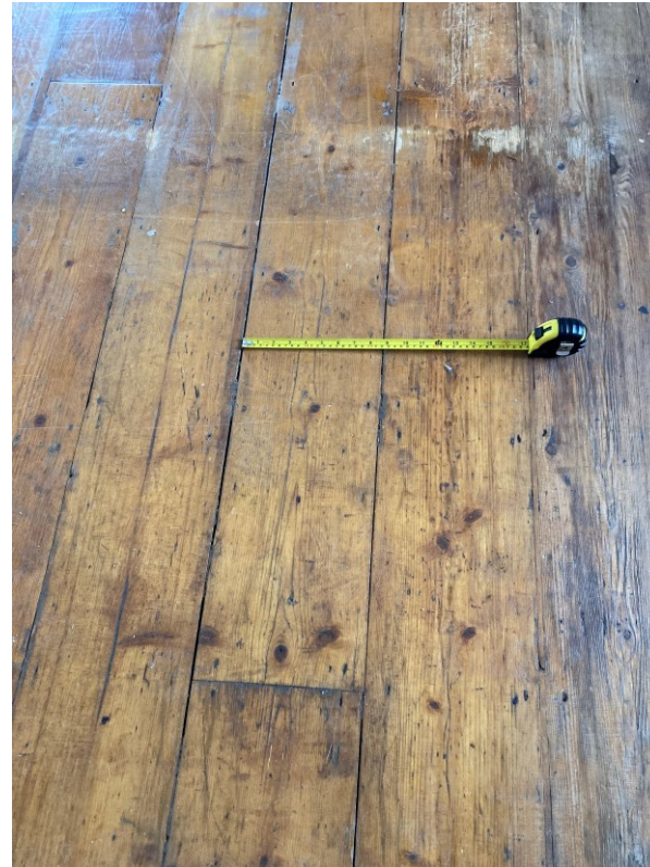
Example- FF Dressing Room, existing floor boards with attractive qualities and suitable for refixing
