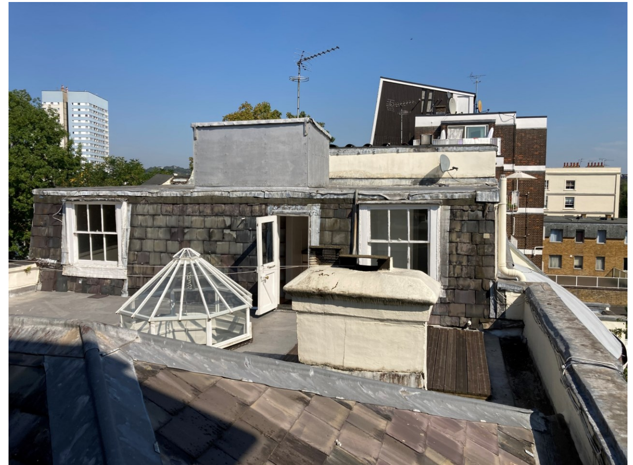
The mansard / second floor accommodation with the pitched roof and flat roof terrace area in the foreground. The large tank housing is central to the flat roof of the mansard.
