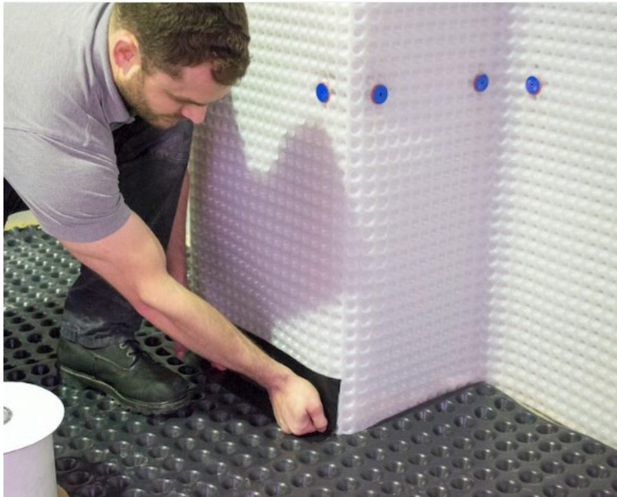
Above- example of the installation of a cavity drainage membrane to floor and walls.
