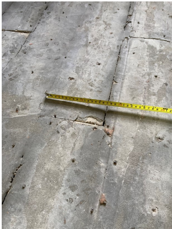
Example- FF bedroom 4, existing floor boards degraded by a application of levelling compounds, not suitable for refixing
