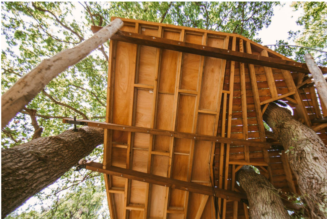
Image showing 2 floating brackets installed on an Oak tree (left tree), allowing 360 degree movement of the tree.
