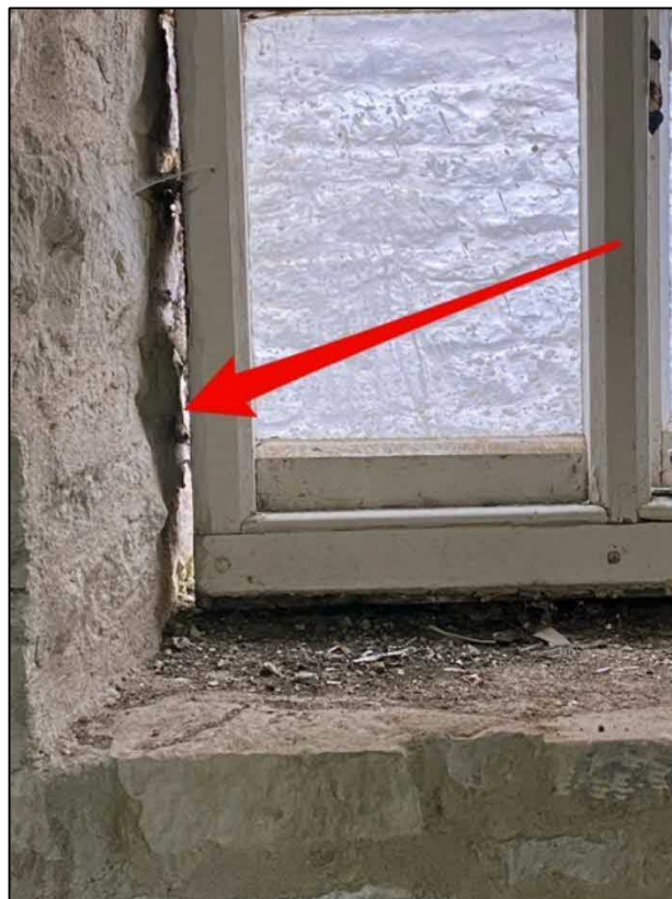
Figure 39 Gaps around window frame
