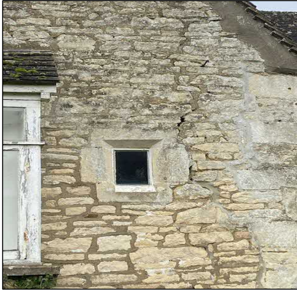
Figure 32 Gaps between stones caused by missing mortar
