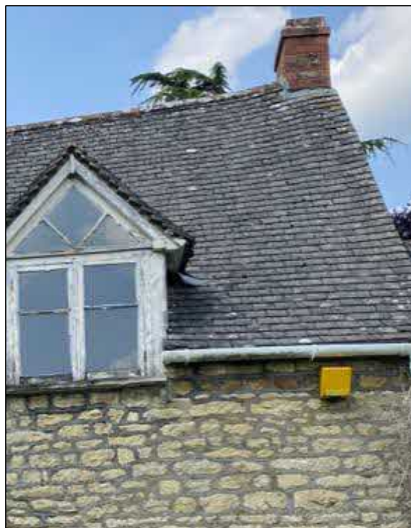
Figure 30 Lead flashing associated with dormer window
