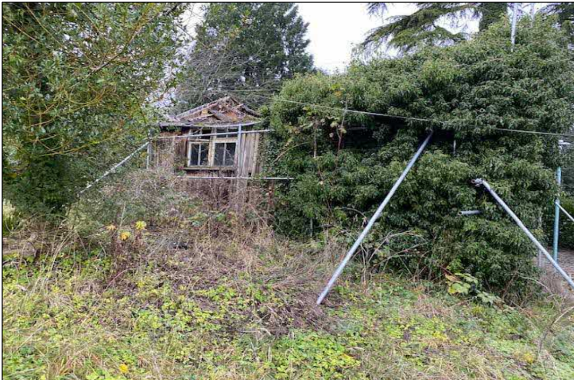
Figure 21 Dilapidated timber shed
