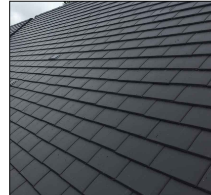
Gray shingles, roof tiles of the existing house to be matched to the proposed building
