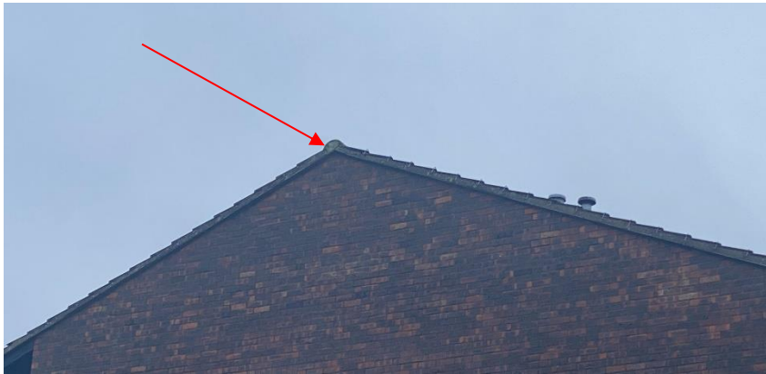
Plate 4.3: Missing mortar on the ridge tile (Northern Elevation)
