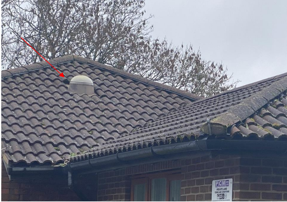
Plate 4.16: Missing Clay Tile Near the Air Chimney (Eastern Elevation)
