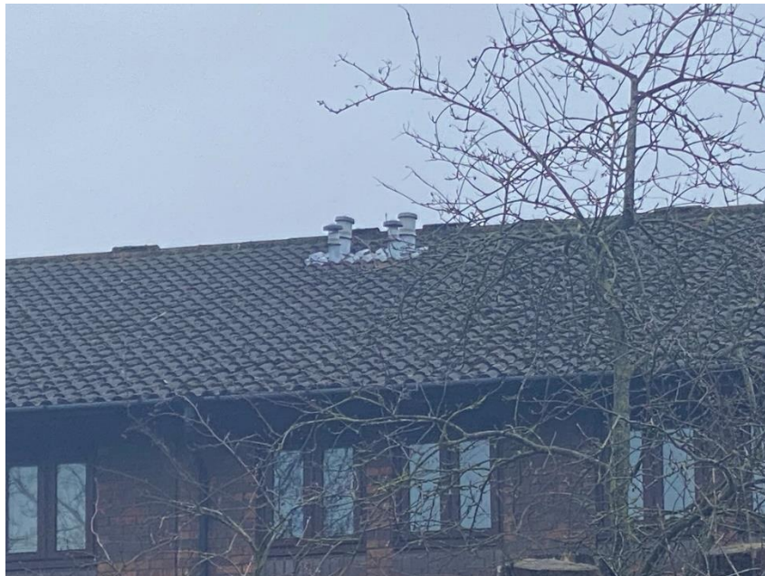
Plate 4.4: Lifted Lead Flashing at the Base of Steel Chimneys (Western Elevation)
