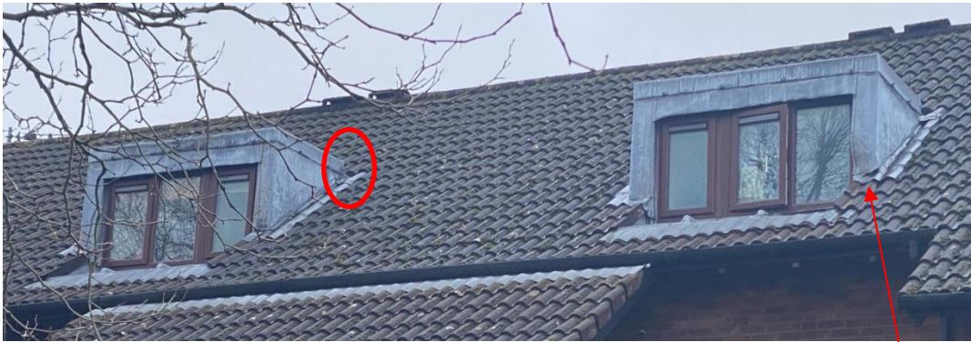
Plate 4.12: Gaps Noted Between Led Flashing and the Roof Tiles (North Elevation)
