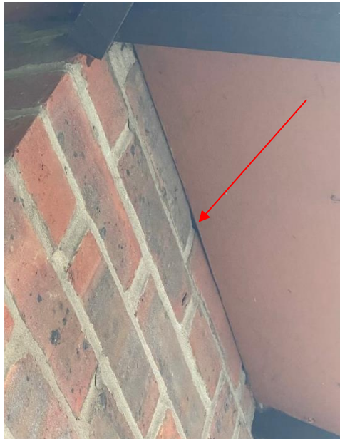
Plate 4.17: Gap Between Soffit Box and the Brick Wall (Southern Elevation)
