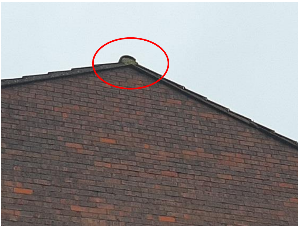
Plate 4.8: Missing Mortar Between Ridge Clay Tiles and Brick Wall (South-eastern Elevation)
