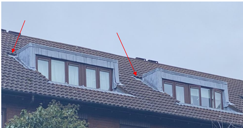
Plate 4.13: Gaps Noted Between Roof Tiles and Led Flashing (Southern Elevation)
