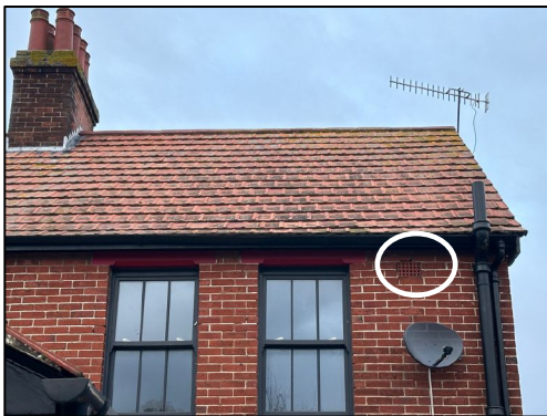
Figure 17 – Location of the vent and gaps close to the satellite disk on the main house
