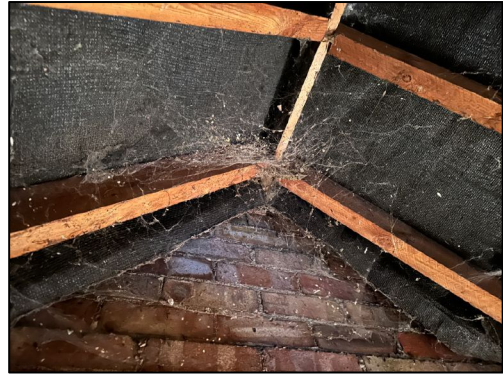
Figure 10 – Level of cobwebbing in the roof framework
