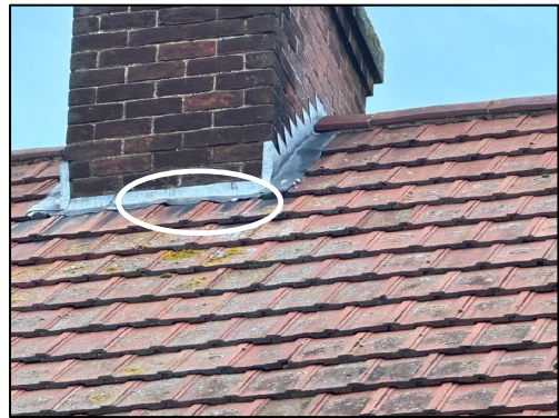
Figure 18 – Slightly lifted area of lead flashing
