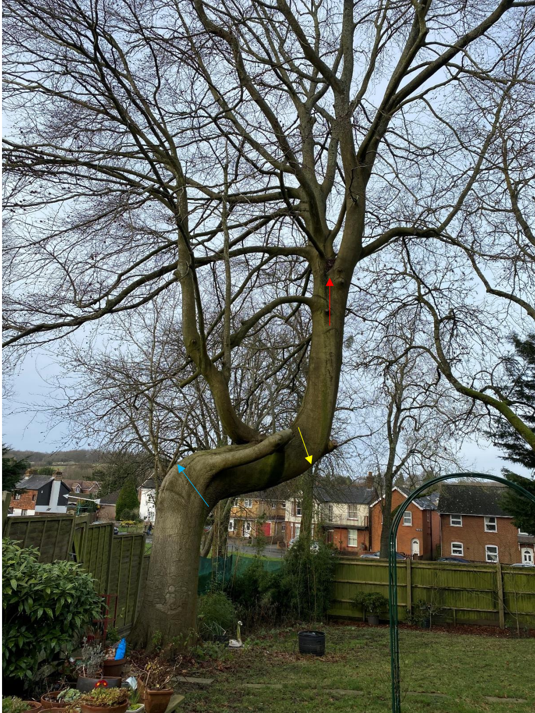
SAL6 T7 beech with included bark union (identified by red arrow), bends in lower stem, exposed bark (identified by yellow arrow) on underside of bend, and cavity on the tension / upper side of the bend (identified by blue arrow).
