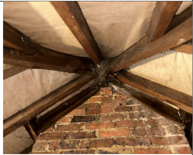
Photograph 4: Dust and cobwebbing around beams
