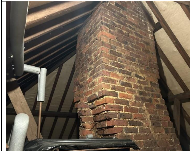
Photograph 3: Void and chimney within
