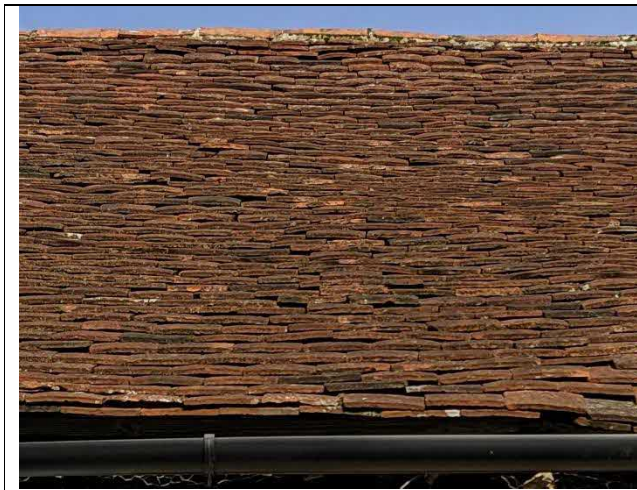
Photograph 3: Gaps beneath roof tiles
