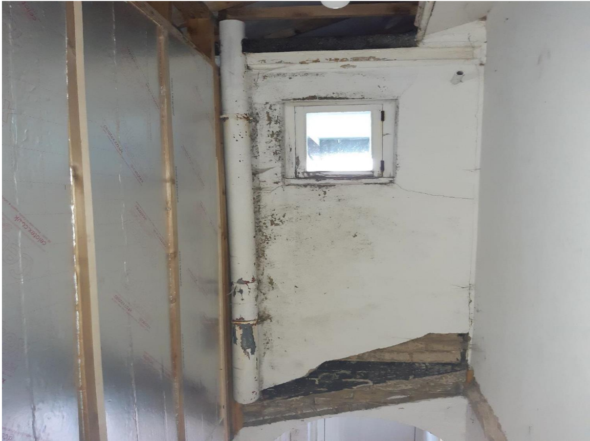
Photograph 2: Interior rear (south) wall of the first floor added storey above the west entrance bay. Note the line of the original single storey roof above the arched entrance and the black bitumen coating to what was the rear of the parapet. The old external downpipe to the added floor is now encased within the building
