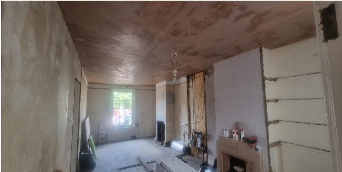
Photograph 8: Interior ground floor looking north. Note the slot in the floorboards marking the line of the former partition and where it terminates. The existing flooring extends continuously to the west indicating the position of the former doorway. Note also the cement rich render exposed to the south of the chimney breast in the rear (dining) room following the removal of shelving. Both chimney breasts were obviously re plastered (or rendered) following insertion of the 20 th century fireplaces.
