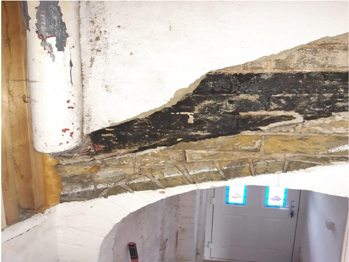
Photograph 3: Detail of the former pitch roof detail over the entrance bay and the rear of the parapet with the later downpipe diverted through the wall above the former roof. Note the thick cement render over the brickwork added to cover up the junction between the different storeys.
