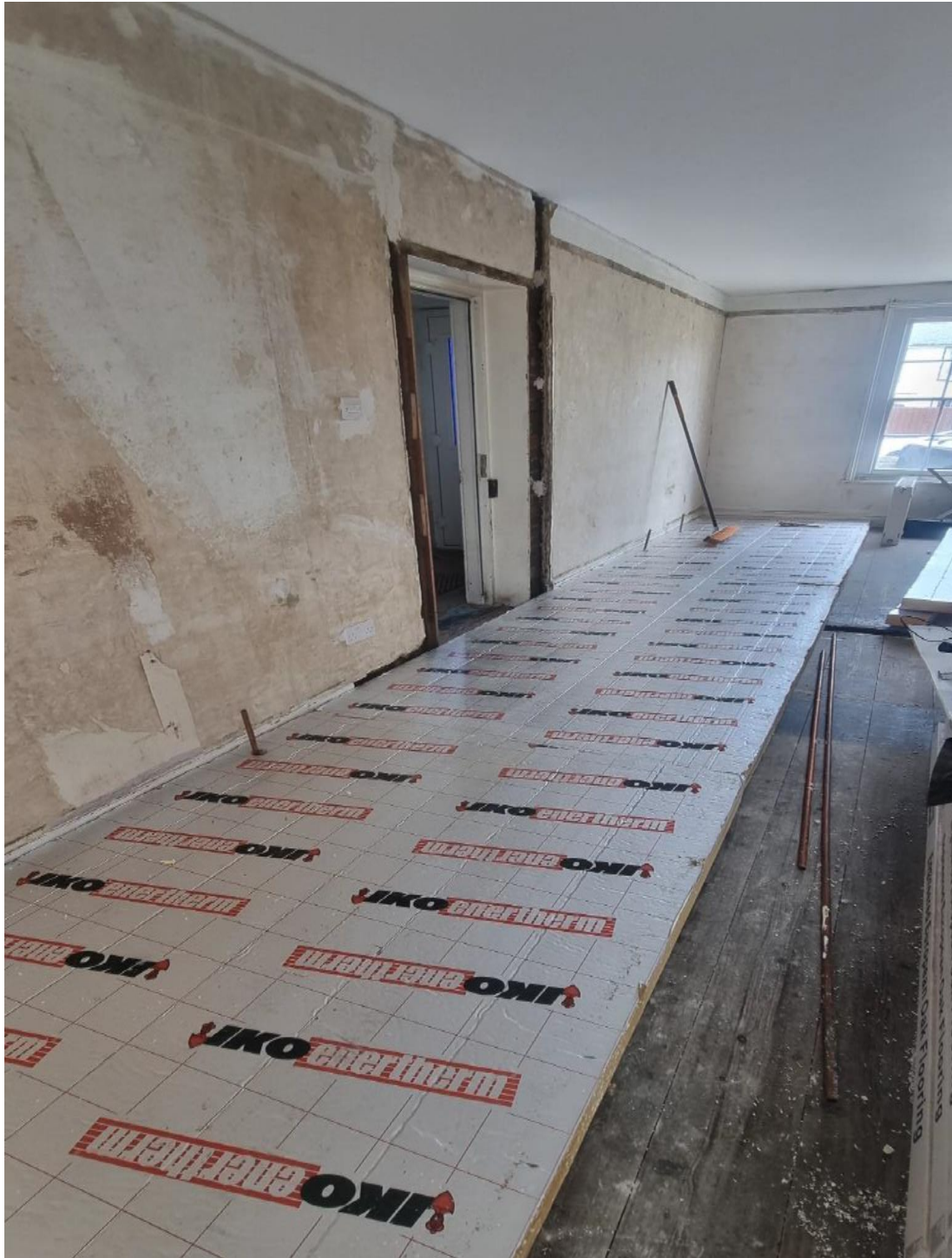
Photograph 5: Interior Ground Floor looking north. Note the line of what was the historic partition to the north of the inserted side entrance. Note also lack of the line of a picture rail above the entrance door and the different line of the vanished picture rail in the rear room. The laminate floor is being laid over the earlier stained floorboards and encasing the existing skirting.
