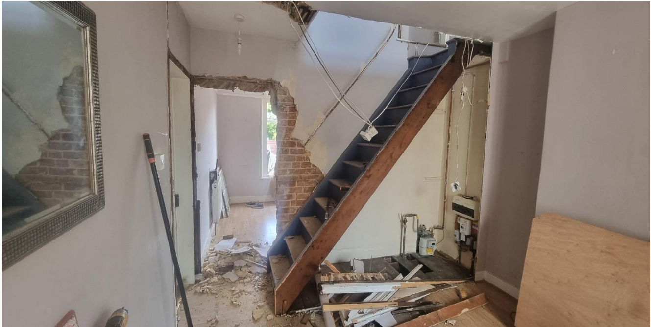
Photograph 11: Interior former stair now removed. Note the steep pitch because it had to be inserted in a restricted space between the new western entrance and the blocked opening at first floor level in order to be able to serve the existing bedroom doorways. The landing is therefore effectively in the form of an enlarged upper step and attached to the restricted area above the former connecting door between the two properties. It could not block the existing opening between the two rooms and it is therefore more akin to a ladder with a closed string and no balustrade, being enclosed between an existing and an inserted partition. The existing partition was brick which is seen exposed in this photograph and the later partition to the south was very thin and timber.
