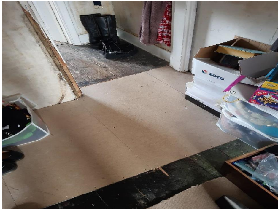
Photograph 9: Interior first floor. Temporary infill of former stair opening. Doorway is the remains of the historic first floor partition space beyond was in the former bedroom now provides access to the bathroom to the west
