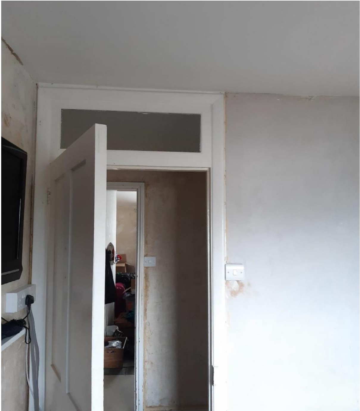
Photograph 10: Interior first floor north bedroom looking south to the new partition attached to the chimney breast with the modern door opening under the glazed transom light. The original partition is beyond leading to the first-floor south bedroom.
