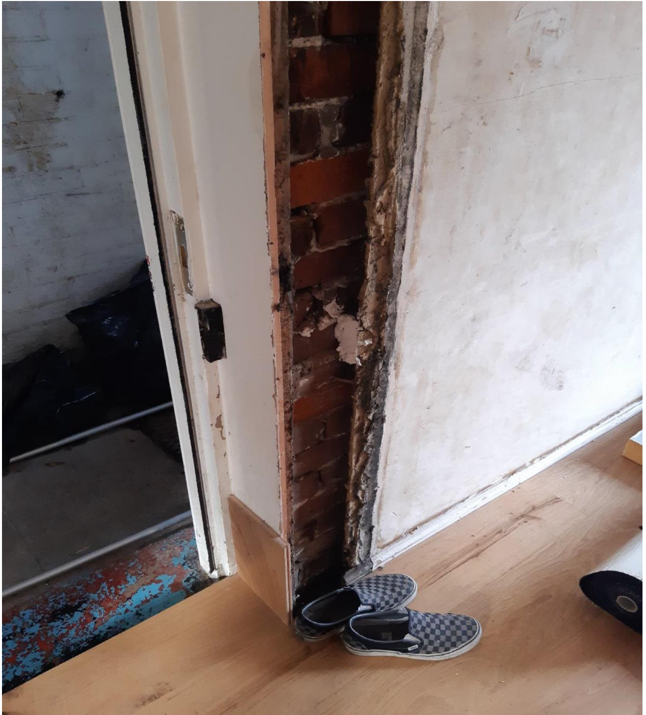
Photograph 6: Ground floor interior north of the side entrance. Note the line of the architrave removed from the door- the original partition did not extend this far- and other evidence shows this was where the door into the north room was sited. Note also the regularity of the exposed lathe ends and the nature of the finishing coat of plaster. Also note the profile of the small section of the skirting above the laminate floor which is not typical mid-19 th form but rather that used from the later 19 th century right up until the mid-20 th and evidence that the room has been refurbished
