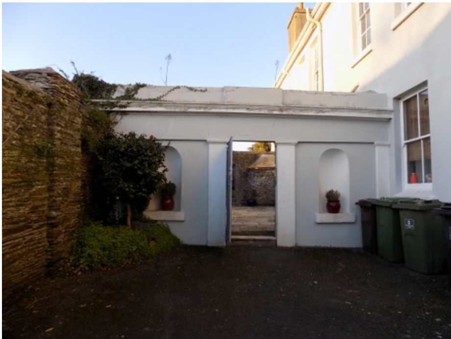
Photo 10. Stucco rendered stone wall with alcoves to inner courtyard to service wing.
